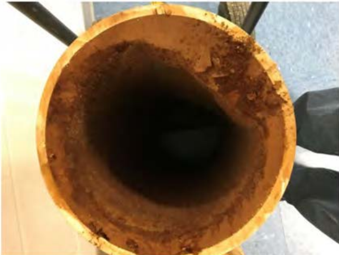
SEWUD-West 12-inch Raw Water Supply Line □ Iron Build-Up (2017)
