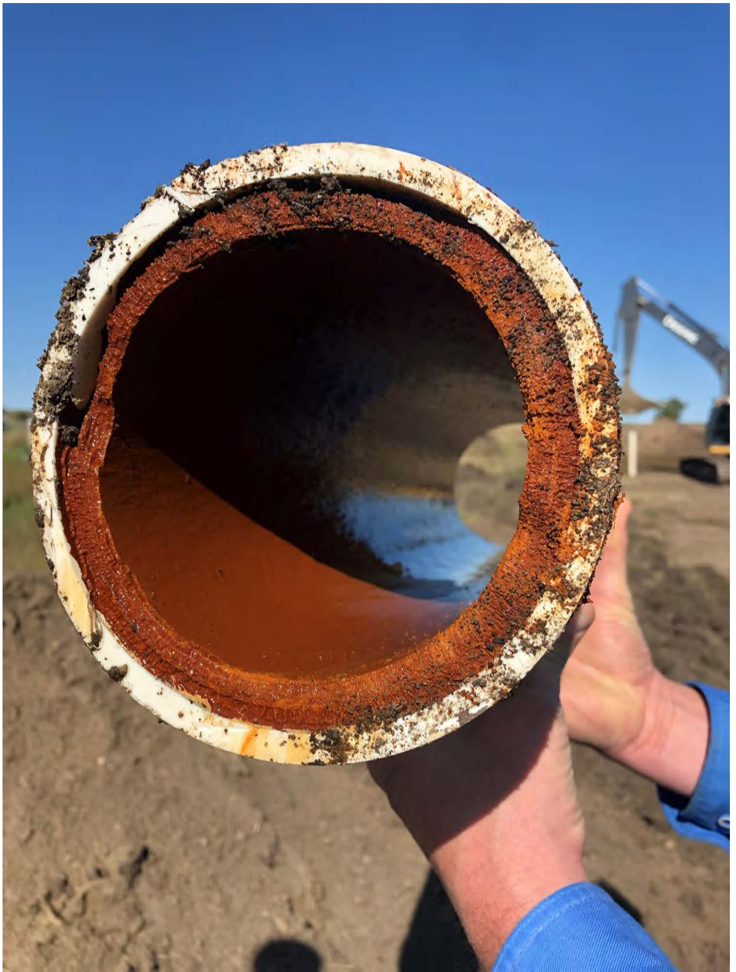
SEWUD-West 6-inch Raw Water Supply Line □ Iron Build-Up (2019)
