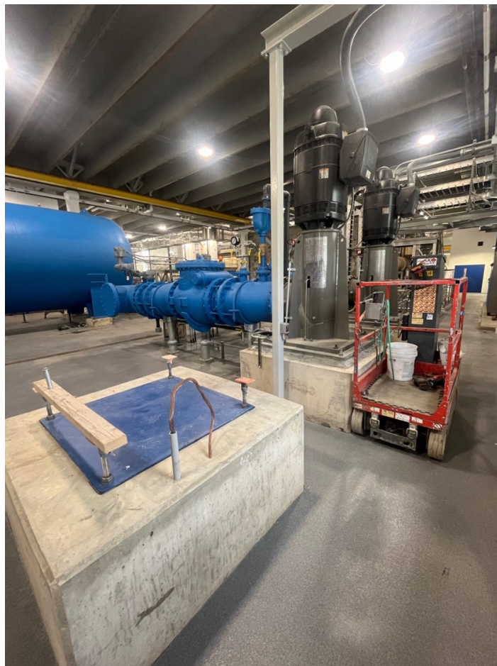
Photo 3: Biota Water Treatment Plant, August 2024
