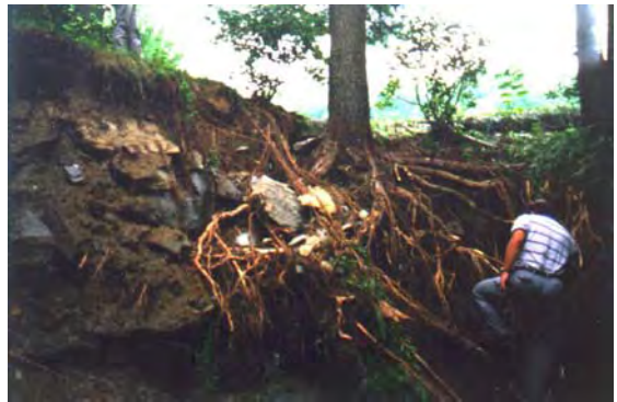
Figure 6. Tree root induced scouring on crest and downstream face of Coffey dam in Kansas.
