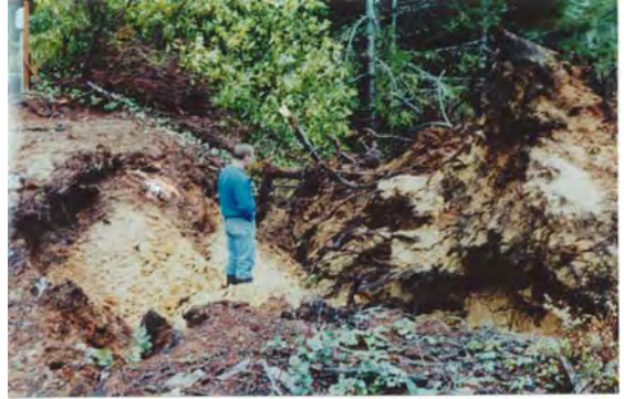
Figure 5. Serious damage by uprooted tree to embankment stability at a dam in Oregon.
