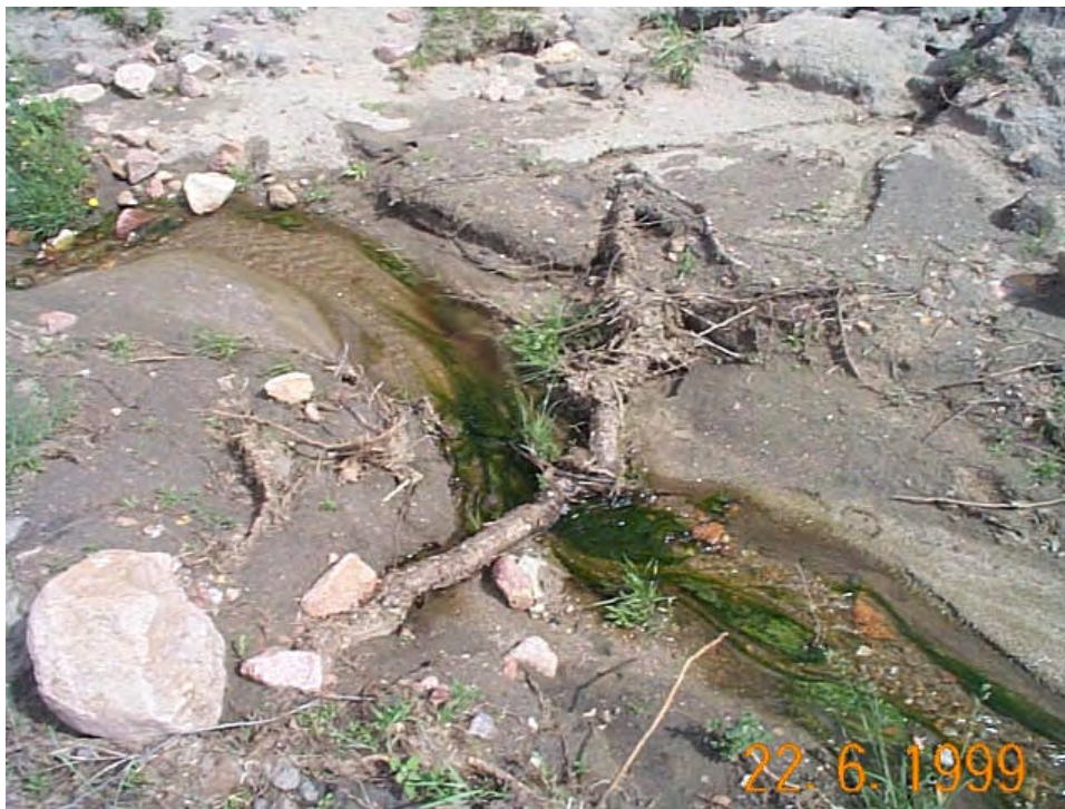
Figure 9. Large pine tree root located in the channel of the breach opening of a failed Air Force Academy waste lagoon pond dam (David Eyre, Senior Civil Engineer, Air Force Academy, Colorado, 1999).
