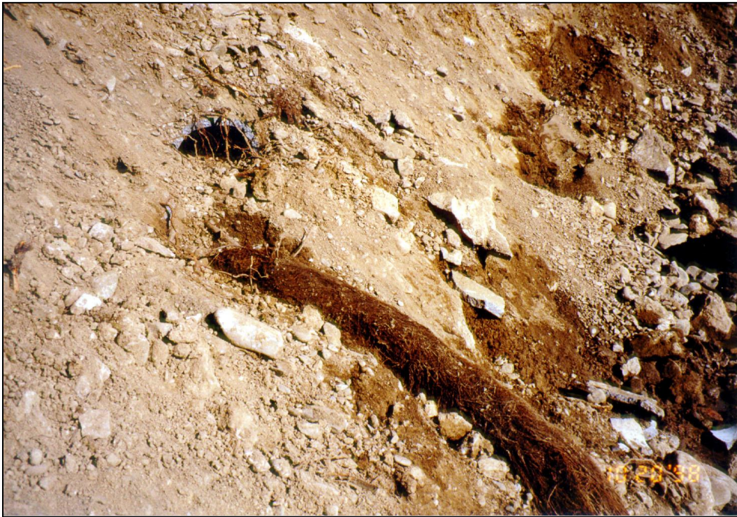
Figure 2-19. During modification of a dam, this toe drain pipe was exposed during excavation. The pipe was completely clogged with the root ball shown in the foreground. It was noted that a tree was growing over the toe drain, and the drain was probably the water source in this arid region of central Oregon.
