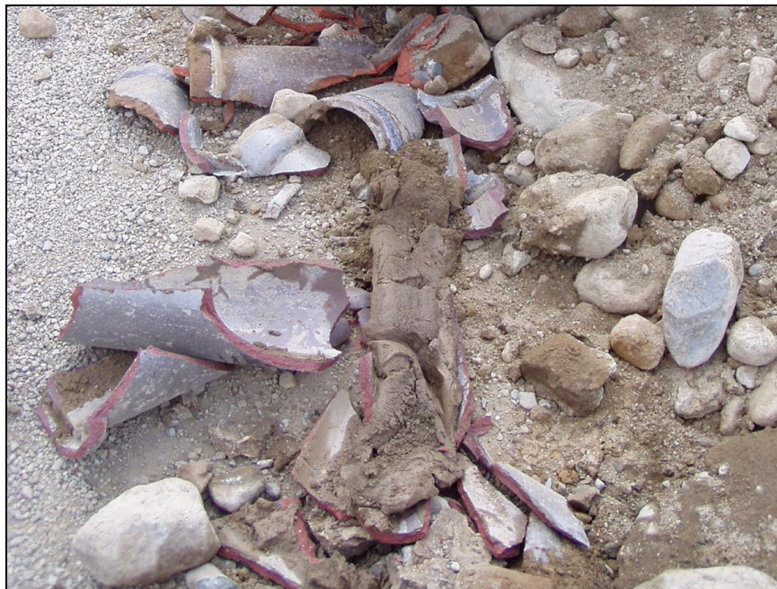
Figure 2-18. Clay tile pipe from 1916 as it was exposed during excavation. Note that the pipe was completely clogged with silt and sand.
