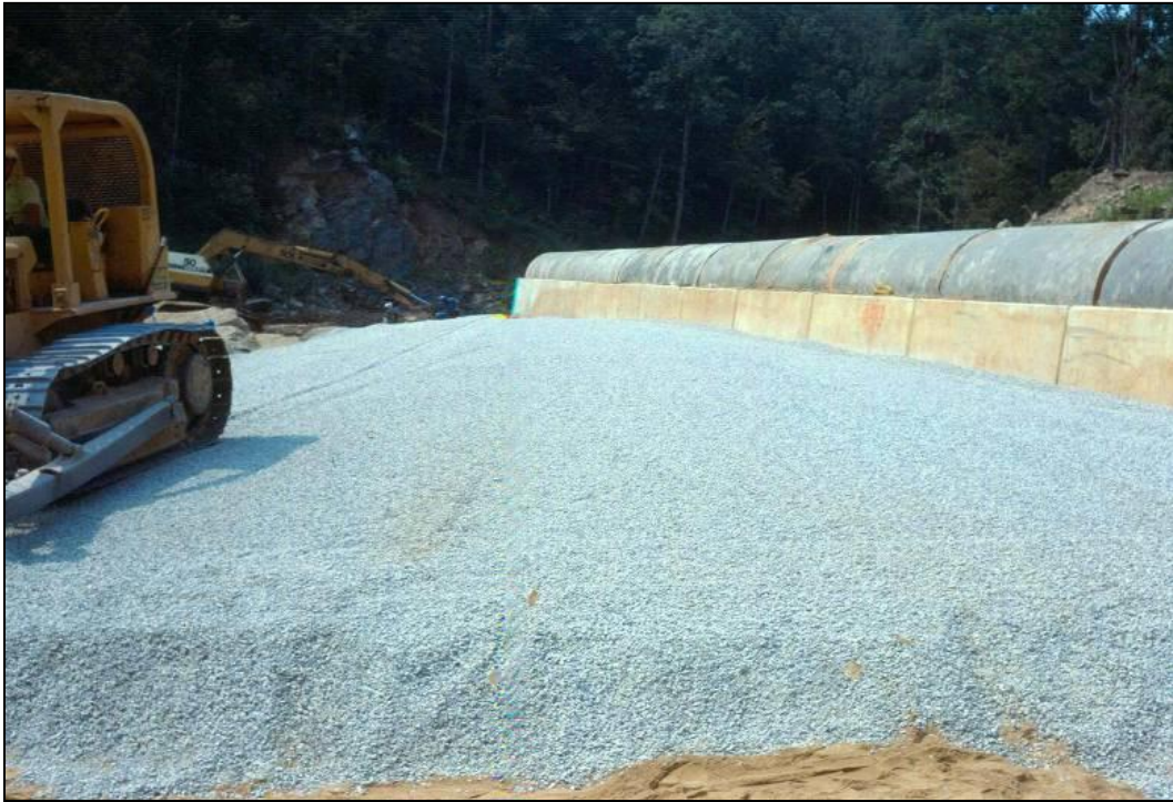
Figure 2-10. Gravel blanket drain being placed over fine filter shown in Figure 2-9. (Photo courtesy of NRCS, Alabama.)
