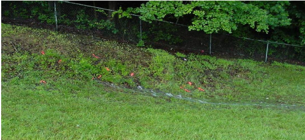
Figure L-26-1. Water discharging in the groin area downstream of an embankment during higher than normal reservoir storage. Seepage was through bedrock in the foundation that was not grouted. A gravel drainage layer was placed over the seepage to provide a controlled outlet. The seepage was not carrying fines, which would have been problematic to deal with because a fine filter would be required to block the fines but a coarse filter was required for capacity. In this case, the gravel layer provided a collector mechanism, with no filtering being required.
