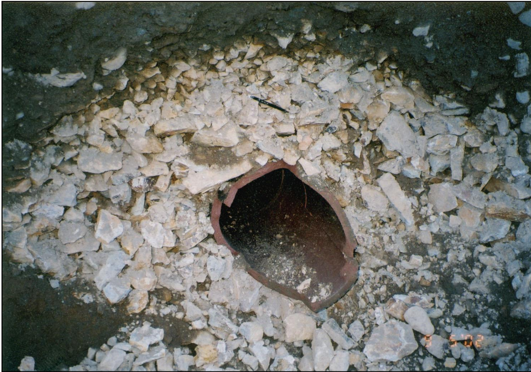
Figure 2-16. Clay tile pipe surrounded by gravel-size material. Note mechanical pencil for scale. Surrounding the gravel is a mixture of silt and sand backfill that does not meet filter criteria for the gravel. Seepage enters the pipe through joints between pipe segments. The silt and sand can erode through the gravel backfill and enter the pipe through the joints.
