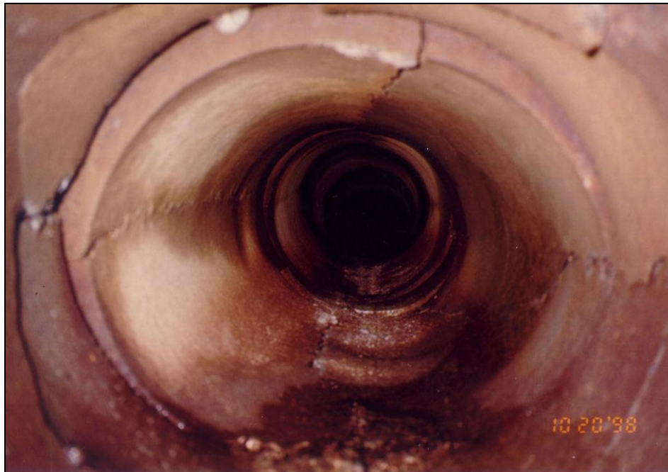
Figure 2-17. Interior view of a reinforced concrete pipe from the 1950s. Note that the pipe is overstressed, and cracks have formed at the crown and spring line. The pipe has also deformed to an oval shape. In the foreground, a joint can be seen and sand that passed through the joint.
