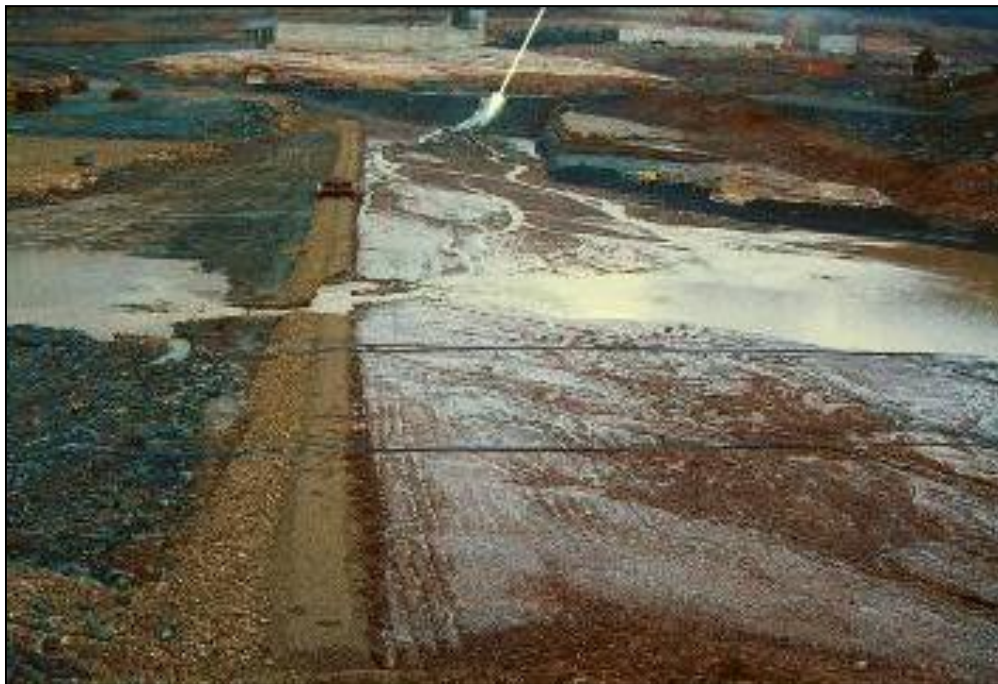
Figure 7-25. Surface water contamination of a chimney filter.
