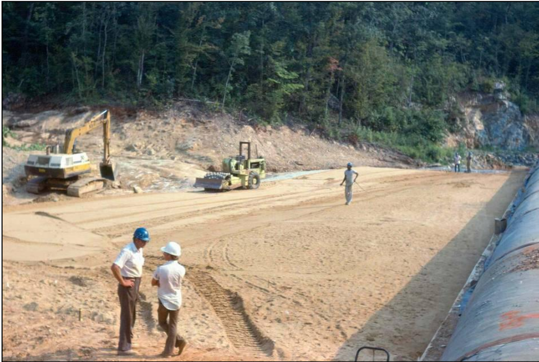
Figure 2-9. Fine filter being placed on the bedrock surface under the downstream shell of an embankment. View is toward downstream toe. Conduit is on the right of photograph. Exposed bedrock not yet covered is in background behind excavator. (Photo courtesy of NRCS, Alabama.)
