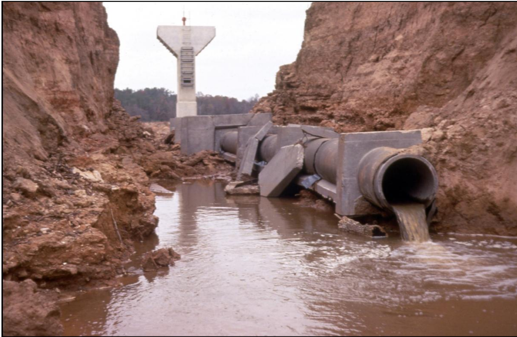
Figure 2-5. Embankment dam breached after piping along the conduit. The view is upstream. Note pre-cast concrete pipe placed on a concrete cradle and the use of seepage collars (Photo credit NRCS).
