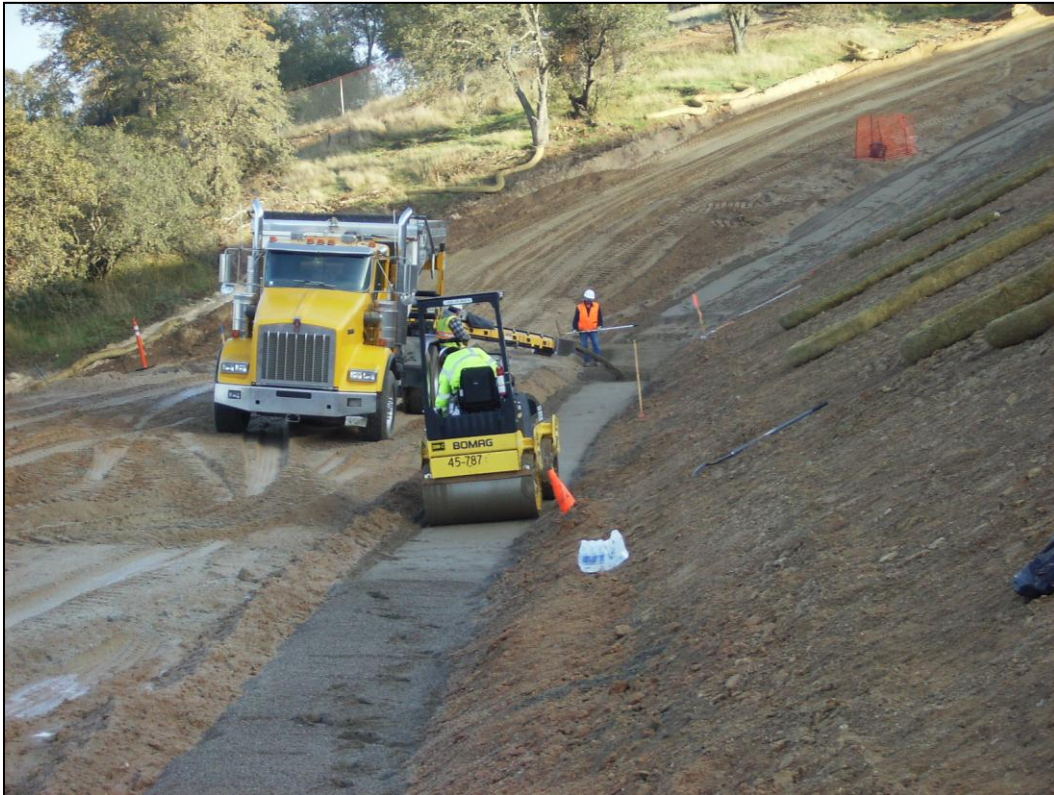
Figure 7-20. Truck conveyor delivering filter sand for the addition of a 4-ft-wide chimney filter to an existing embankment. Note that the material is uniformly placed from the conveyor, and no leveling is required. Dynamic compaction is provided by the roller shown in the foreground.
