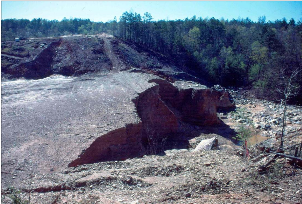
Figure E-2. View toward left abutment. This 50-ft-wide section of the dike overtopped and eroded a portion of the dike.
