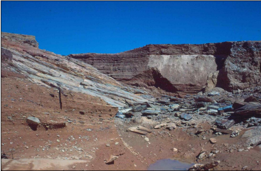
Figure E-3. Breach in left abutment viewed in upstream direction. Right abutment is to left foreground. Overtopping flow washed the embankment and overburden down to clean rock.
