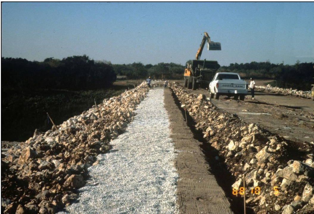
Figure 2-4. Multiple zone chimney filter being constructed in zoned dam by concurrent method of construction.
