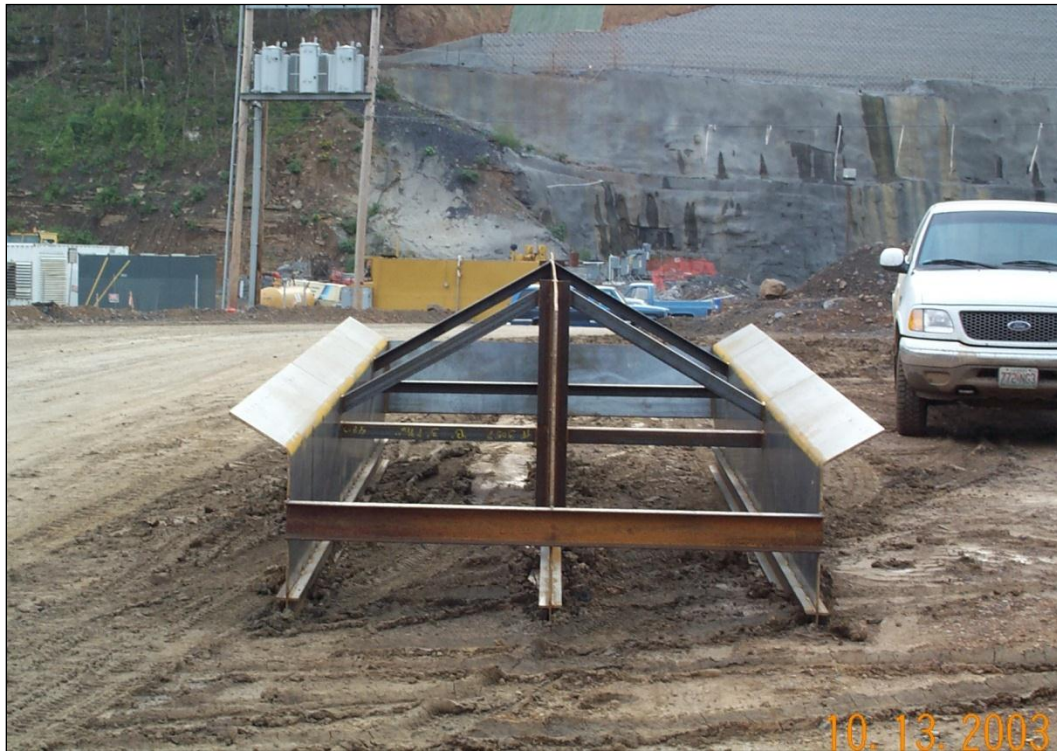
Figure 7-15. Double-bin spreader box.
