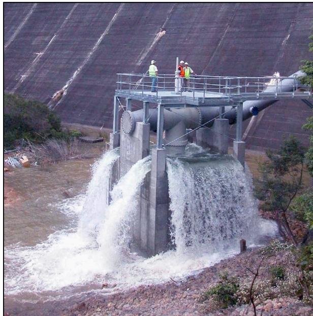
Figure 90. —Submerged discharge valve well for a manually activated 44-inch diameter valve.
