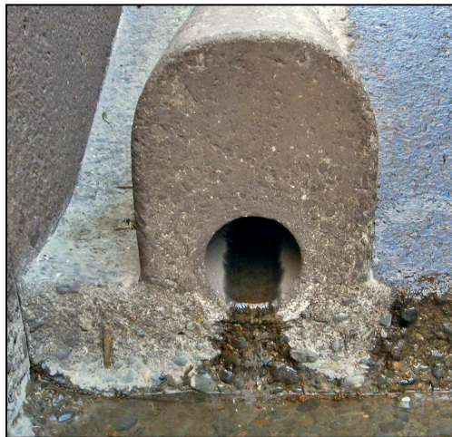
Figure 21. —Looking upstream at a chute block located at the upstream entrance of a stilling basin. A structural underdrain exits from the downstream face of the chute block.
