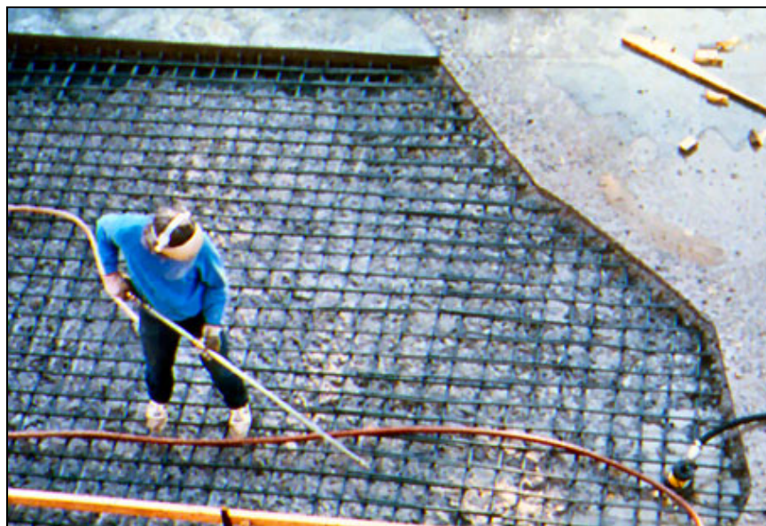
Figure 172. —Blowing compressed air over the surface of the concrete to remove excess moisture.
