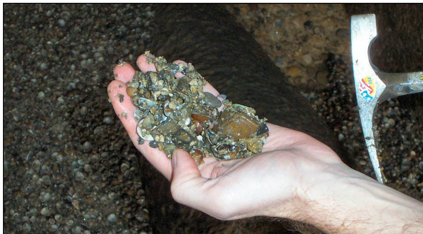
Figure 148. —Eroded concrete caused by abrasion.
