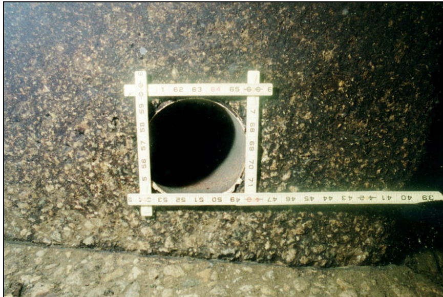
Figure A-107. —Typical condition of drain outfall in downstream face of outlet works stilling basin chute block. Note minor damage to exposed edge of PVC drainpipe likely due to movement of material in basin during releases.
