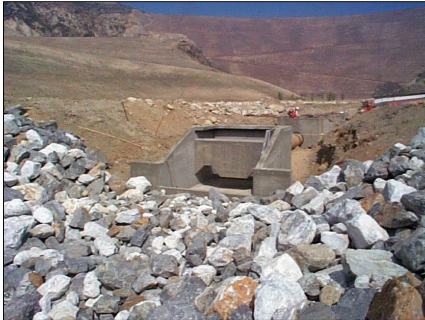
Figure A-92.—Downstream end with impact type energy dissipator (dry).
