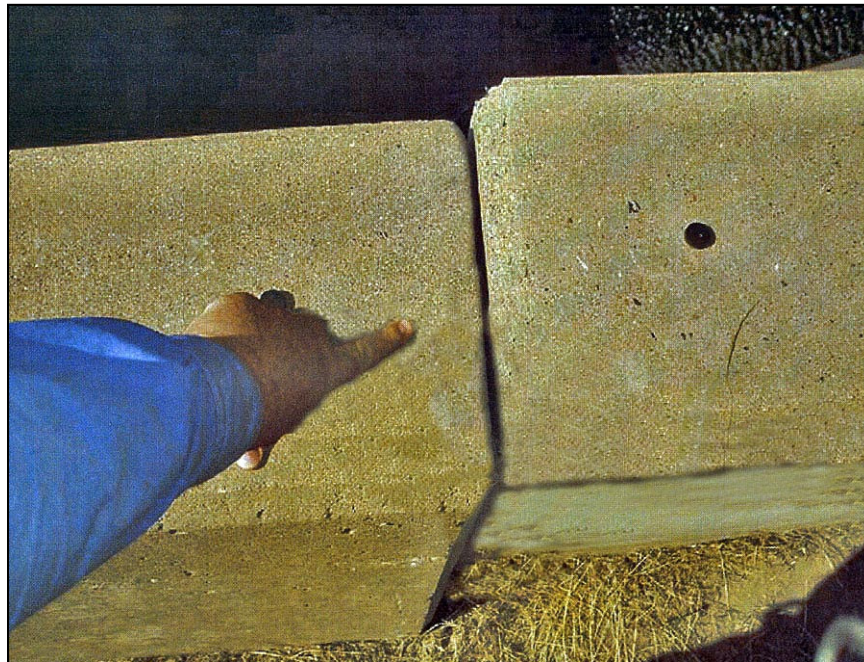
Figure 152. —This vertical wall joint has experienced a 2-inch offset.
