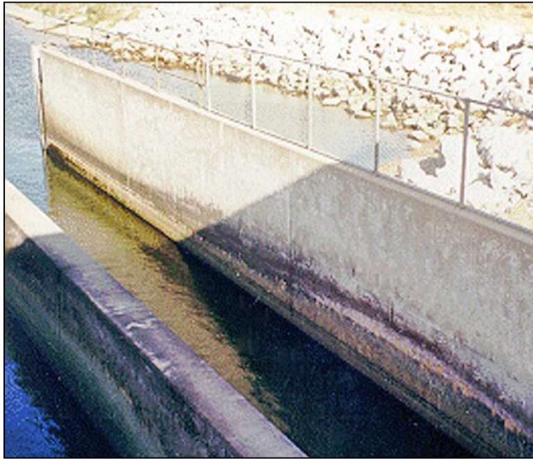
Figure A-120. —Close-up of right wall of river outlet works stilling basin. Arrows denote area of staining from hydraulic jump which roughly corresponds to area with exposed reinforcing steel in floor.
