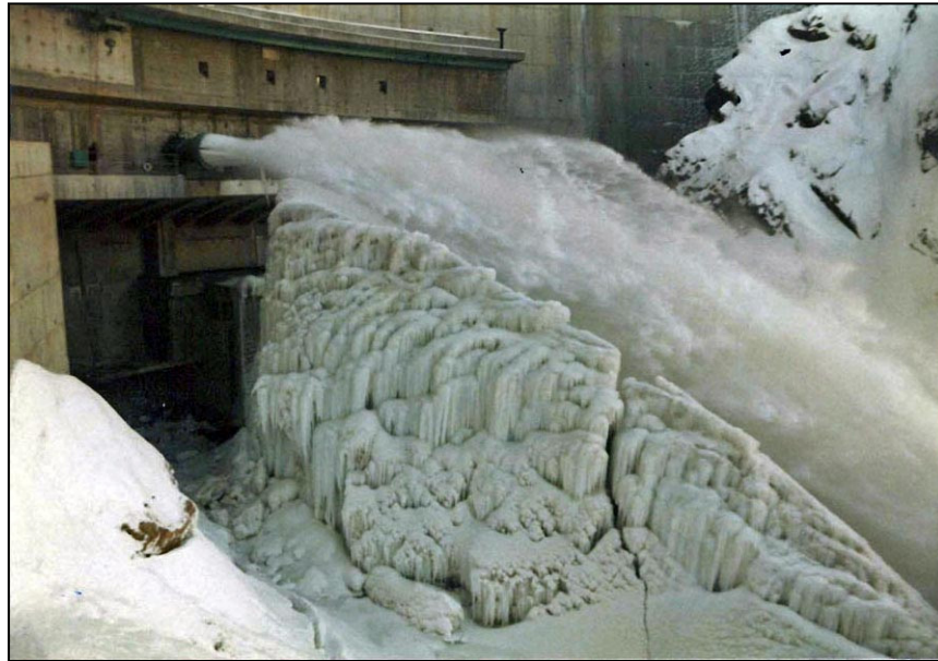
Figure 76. —Ice build-up under 48-inch diameter hooded fixed-cone valves. Ice has built to the elevation of the bottom of the valve operating deck, approximately 60 feet above streambed. Photo courtesy of Denver Water.
