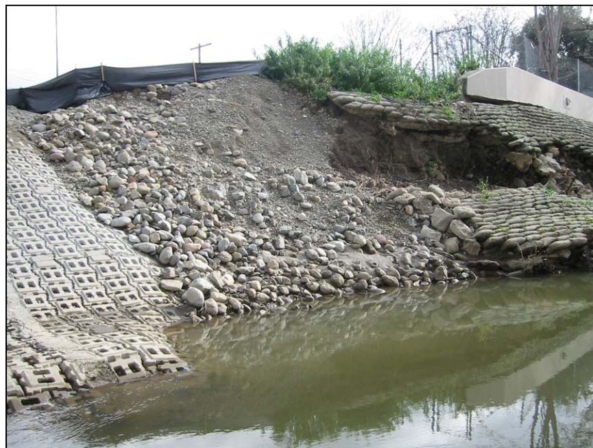
Figure A-30.—Eroded upstream bank.
