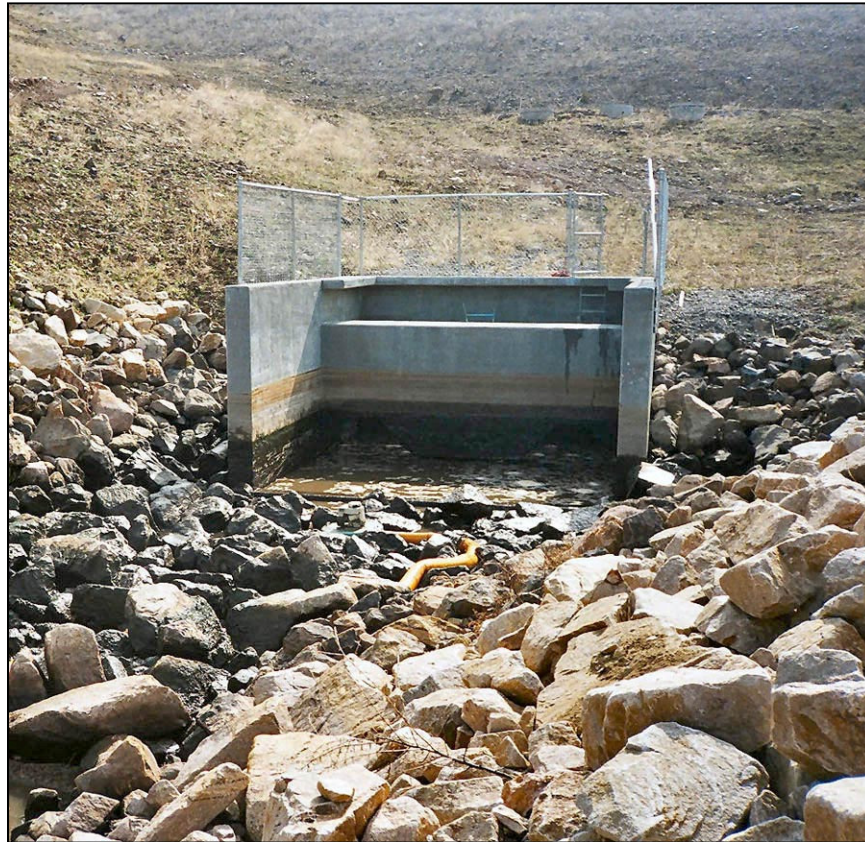
Figure 125. —Transitional riprap apron downstream for a type VI stilling basin to prevent scour.
