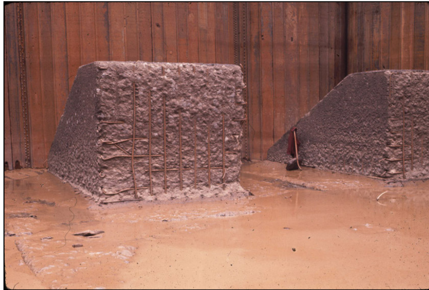
Figure A-39. —Baffle pier damaged by abrasion erosion.
