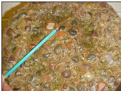
Figure 177.—Minor abrasion erosion damage.
