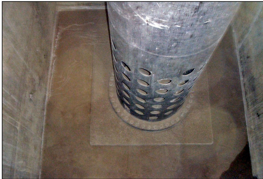
Figure 9. —This 48-inch diameter perforated steel discharge pipe is located downstream of the sleeve valve in a stilling well. The 72 6-inch diameter openings are provided to more evenly distribute the flow from the sleeve valve into the well. The stilling well dissipates any remaining head after the sleeve valve and releases water into the downstream chute without any spray that may cause icing.
