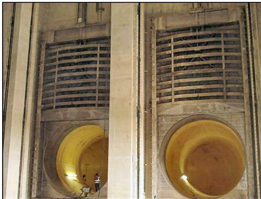
Figure 106. —Installation of large fabricated slide gates. Photo courtesy of Rodney Hunt Corporation.
