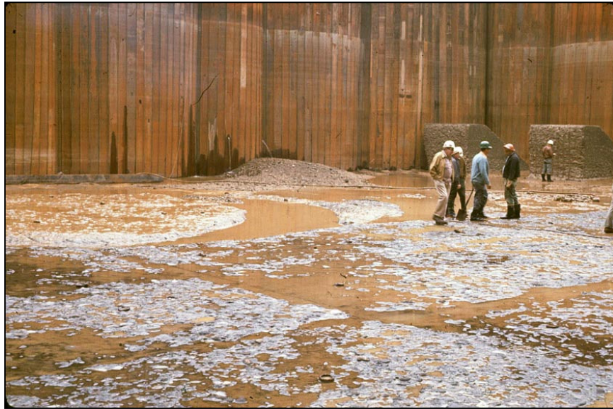
Figure A-37.—Abrasion erosion of the stilling basin slab.
