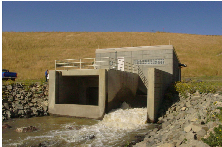
Figure A-23. —View of 18-inch diameter jet-flow gate discharging at about 50 to 70 ft 3 /s (near maximum discharge capacity).
