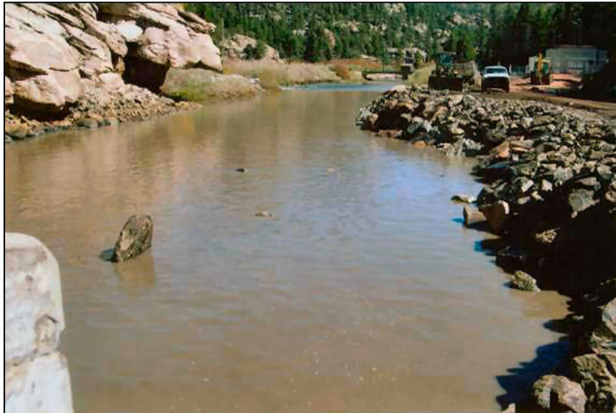
Figure 84. —Erosion of riprap downstream from a 48-inch diameter hooded fixed-cone valve. Photo courtesy of URS Corporation and Denver Water Board.
