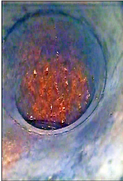
Figure A-108. —View of the first bend inside Underdrain No. 1 (rightmost drain) in the outlet works stilling basin. Image was taken from pipe inspection video.
