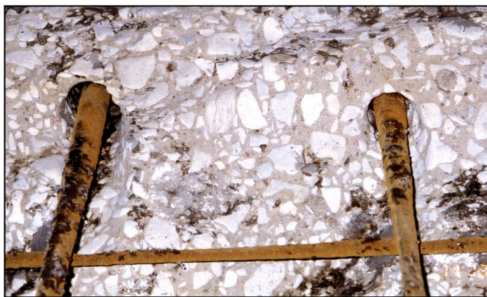
Figure A-122. —Vibration caused the conical openings around the portion of bars remaining in concrete.
