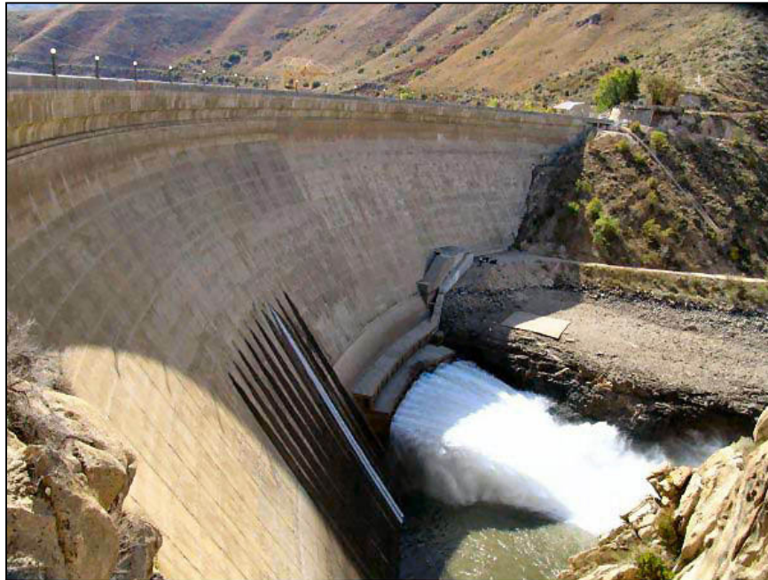
Figure 110.—Ten clamshell gates operating fully open.
