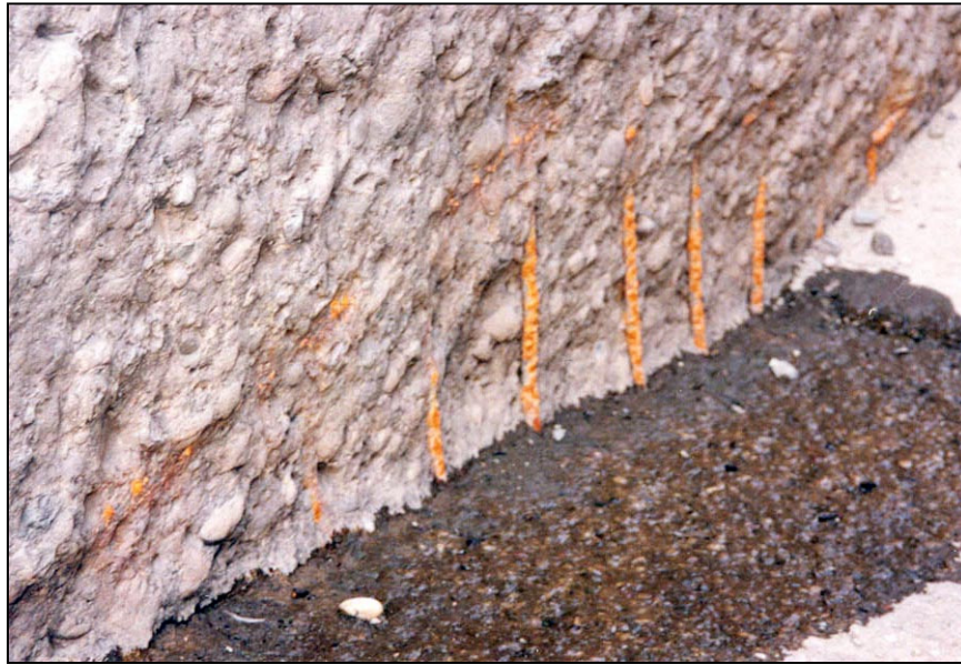
Figure A-69.—Damage to splitter wall.
