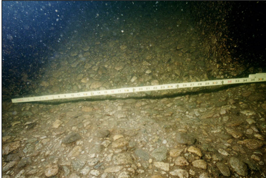
Figure A-115. —Localized erosion between two chute blocks in the outlet works left bay. Note that the ruler is resting on concrete at each chute block and spanning (about 2½ inches above concrete) eroded area in the floor.
