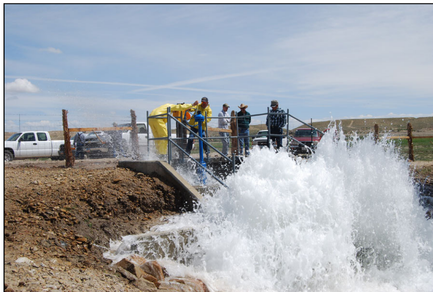
Figure 54. —The end of this outlet conduit was constructed too close to the vertical hanging baffle resulting in intense sprayback.
