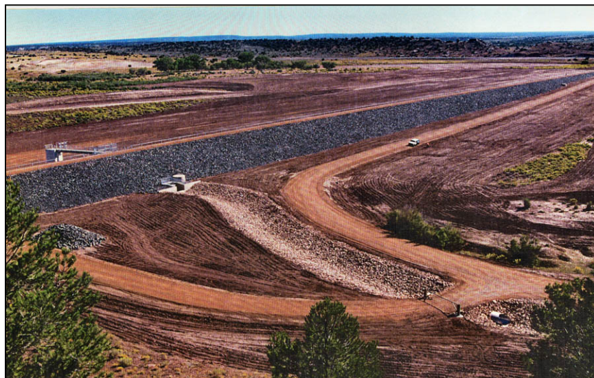
Figure A-25. —Overall view of completed dam modifications from downstream right abutment. The outlet works stilling basin is located in the left center of the figure.
