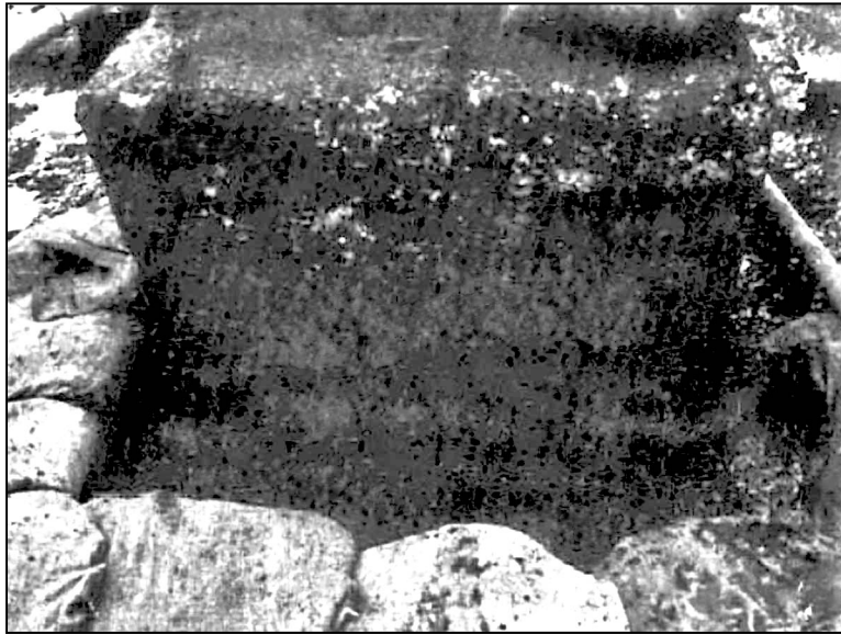
Exposed reinforcement at base of baffle
