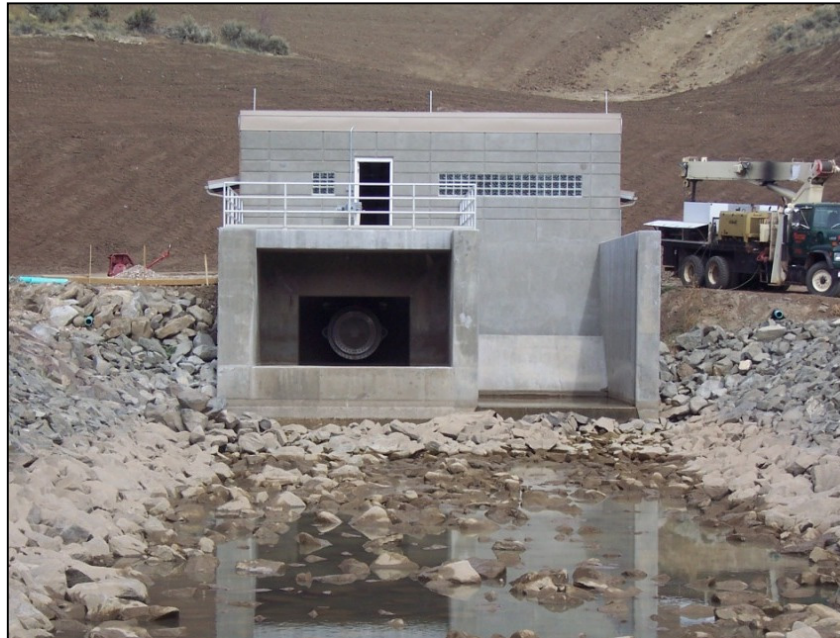
Figure A-19. —View of the completed energy dissipation structure for Elkhead Creek Dam with 42-inch diameter fixed-cone valve in background.
