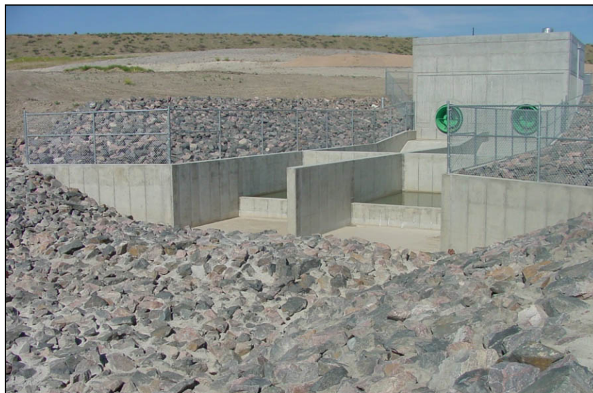
Figure A-97. —View of completed stilling basin for the new outlet works at the stream release facility at Standley Lake Dam.
