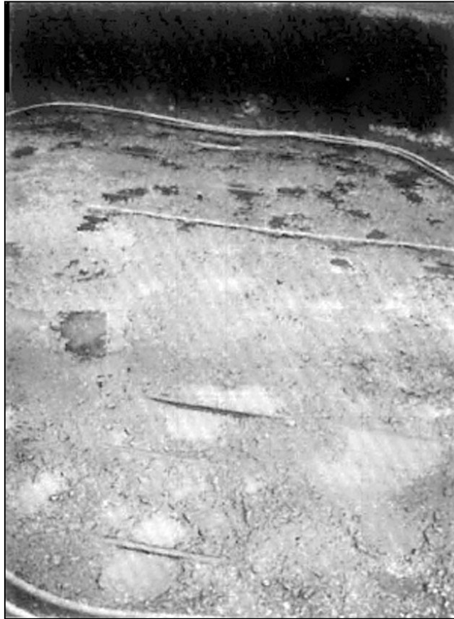
Figure A-8. —Exposed reinforcement in the stilling basin downstream of the baffles.
