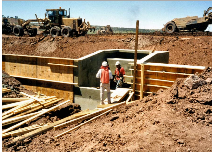
Figure A-26. —Construction crew installing forms for concrete placement of the stilling basin wingwalls.
