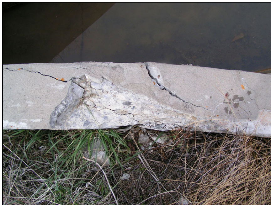
Figure A-57. —Deflection in left wall of dissipator.
