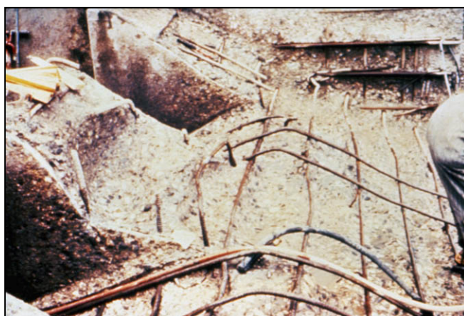
Figure 178.—Severe abrasion erosion damage.
