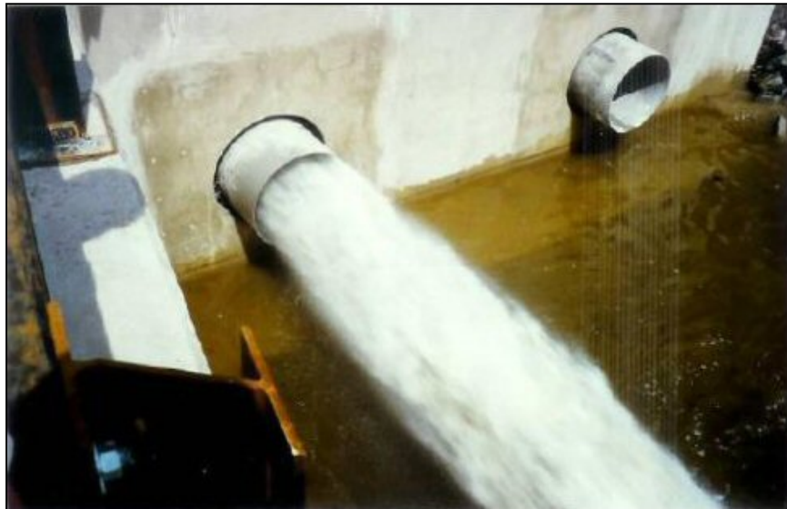
Figure 99. —Jet-flow gate at full opening. Photo courtesy of URS Corporation.
