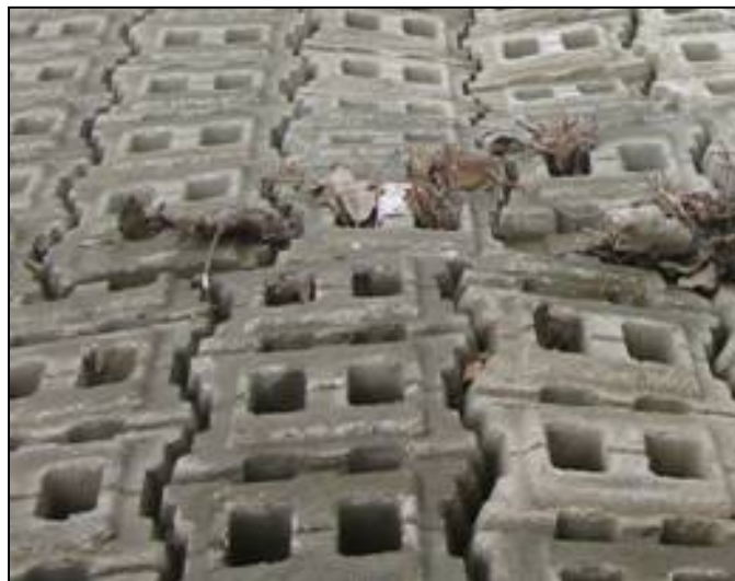
Figure A-33.—Abraded concrete block surfaces.
