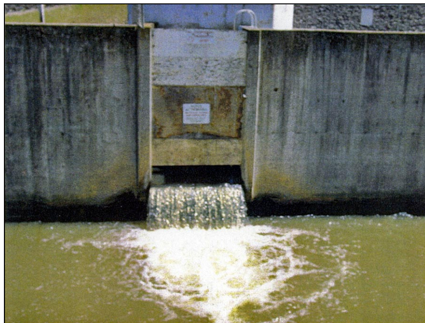
Figure A-5.—Outlet works discharge enters the spillway stilling basin through an opening in the right wall.
