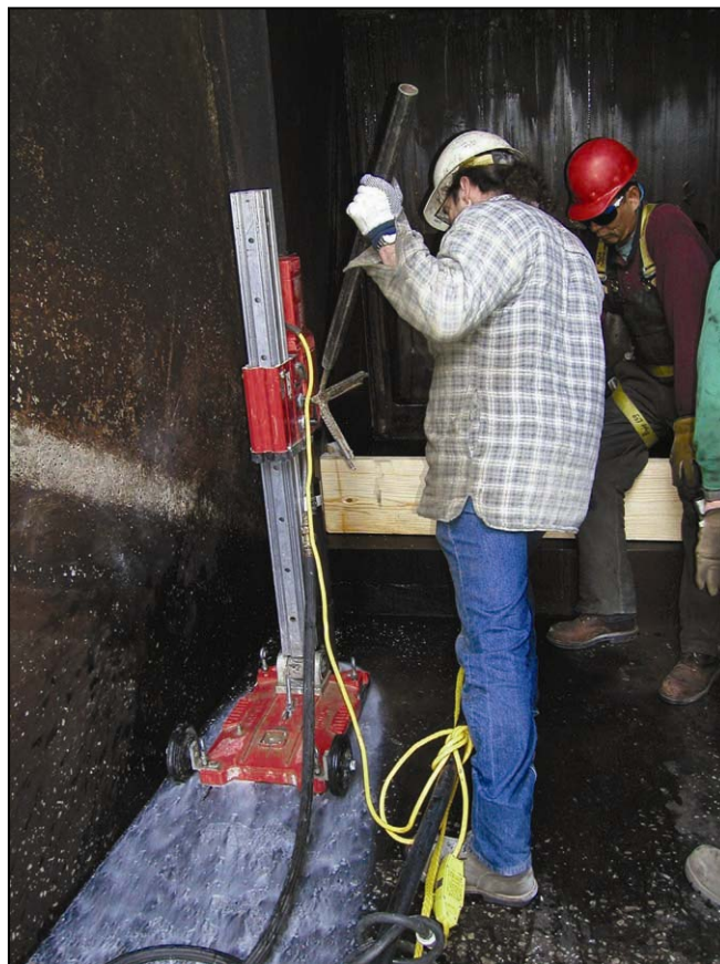
Figure A-126. —Drill crew drilling a hole in right bay of stilling basin.
