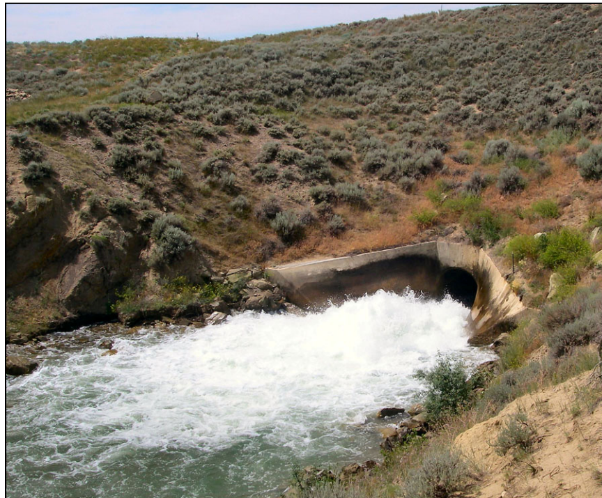
Figure 71. —7.5-foot horseshoe conduit discharging into an outlet expansion with a depressed floor. Downstream channel armoring has also been provided.
