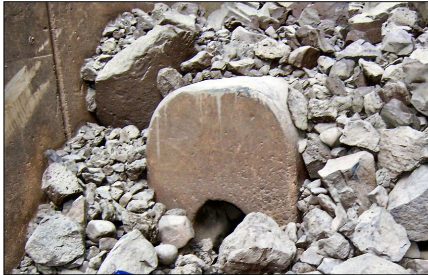
Figure 153. —Debris deposited around a chute block.
