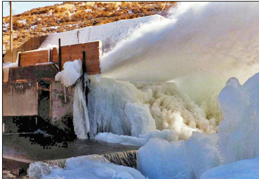
Figure A-46. —Operation of the flip bucket caused significant icing due to water vapor.
