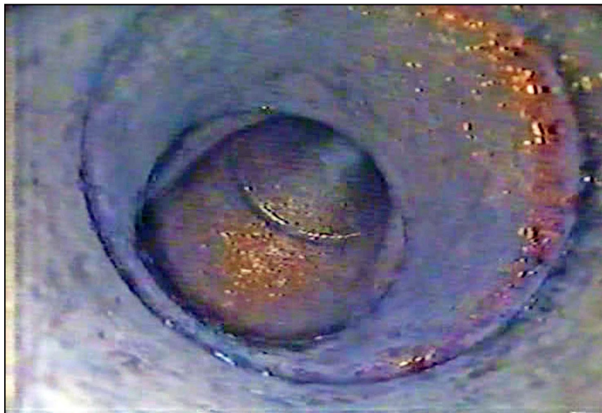
Figure A-109. —View looking vertically downward at the second bend inside Underdrain No. 1 (rightmost drain) in the outlet works stilling basin.
