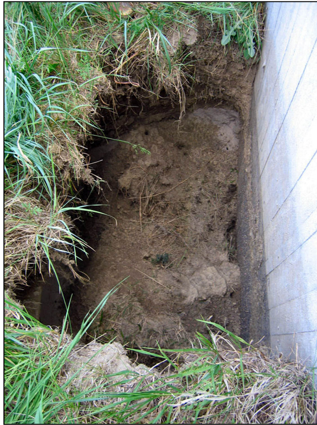
Figure 154. —A sinkhole developed next to this basin wall indicating internal erosion of foundation materials was occurring.
