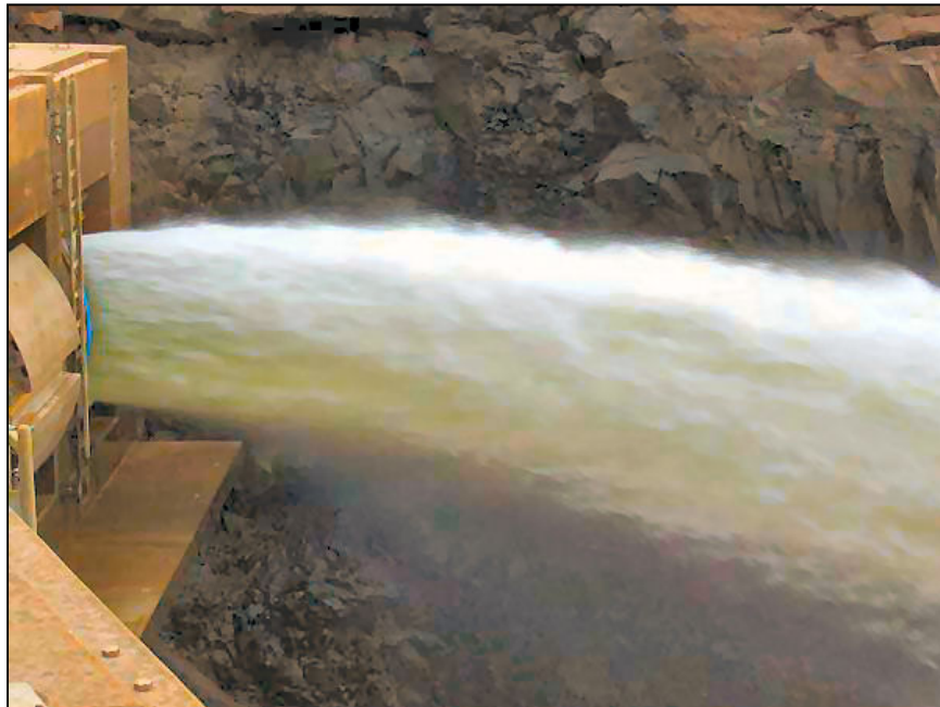
Figure 109. —68-inch diameter clamshell gate at 100-percent open.
