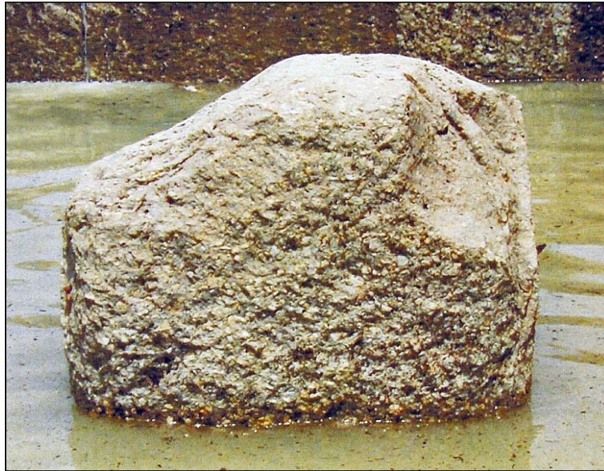
Figure 169. —This baffle block has experienced impact damage resulting from an object in the flow.
