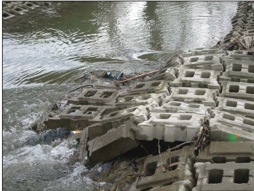
Figure A-32.—Uplifted blocks with loss of granular filter material.
