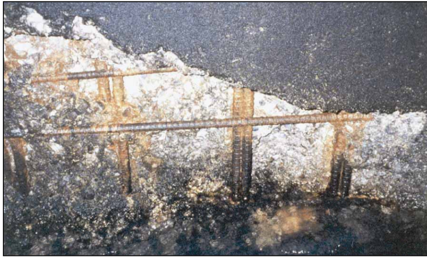
Figure 170. —Chemical attack is often characterized by surface disintegration and spalling.
