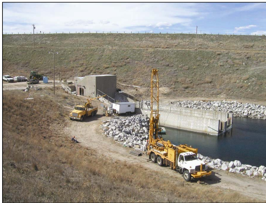
Figure A-124. —River outlet works stilling basin and control house at Virginia Smith Dam.
