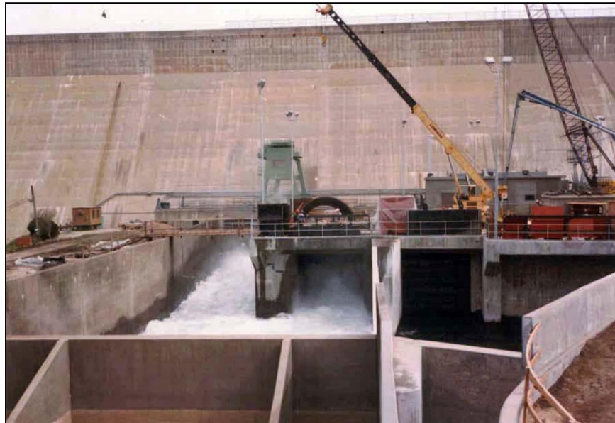
Figure 78. —Discharge from a 96-inch diameter hollow-jet valve on the left (looking upstream) and a 108-inch diameter fixed-cone valve on the right. The discharge from the fixed-cone valve is very calm after passing through the two stage chamber, the spray seen is inside the 2nd stage of the chamber. However, a wave suppressor is required as seen at the bottom left of the figure.
