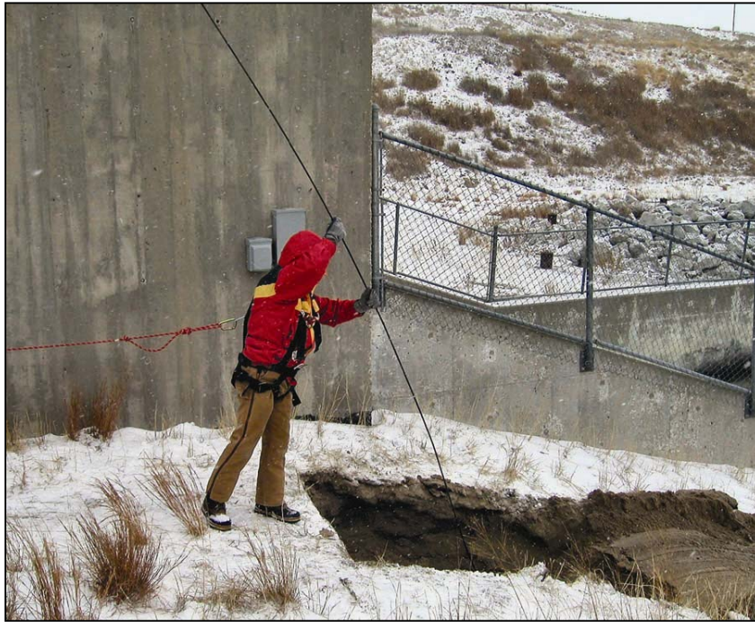
Figure A-125. —The depression is being probed to determine its depth.
