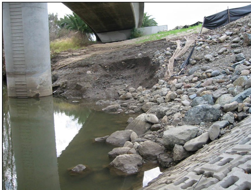
Figure A-31.—Uplifted CCM mats near the bridge pier.
