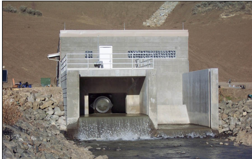
Figure A-21. —View of 42-inch diameter fixed-cone valve under low flow conditions.
