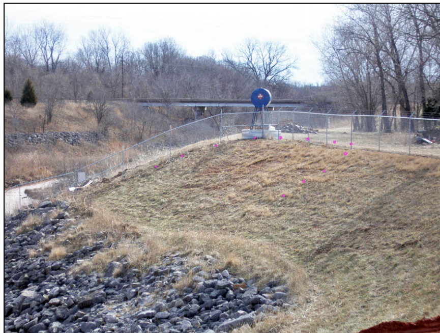
Figure A-63. —Shortly after unwatering, an excavated slope downstream and to the right of the stilling basin was observed to be experiencing cracking and developing a slump. There are pink flags marking the edge of the slump area.
