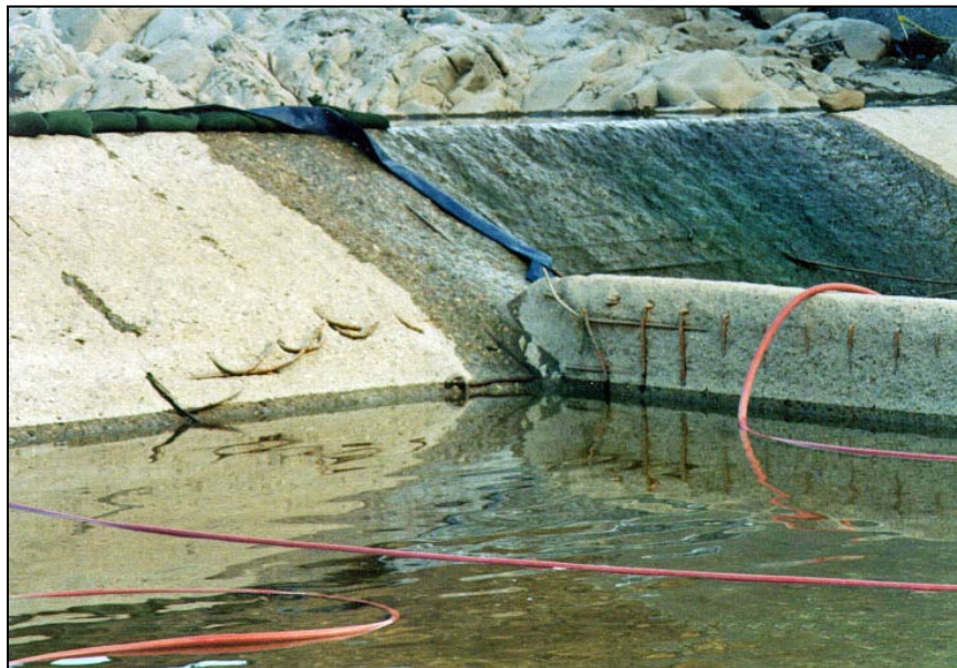
Figure A-70.—Damage to dentate sill.
