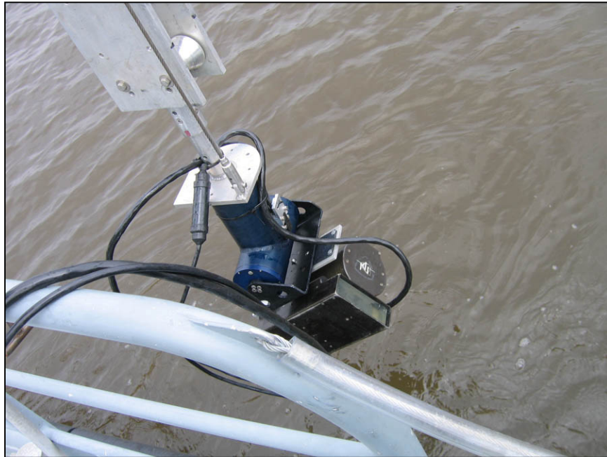
Figure 163. —Acoustical imaging camera mounted with pan and tilt mechanism.
