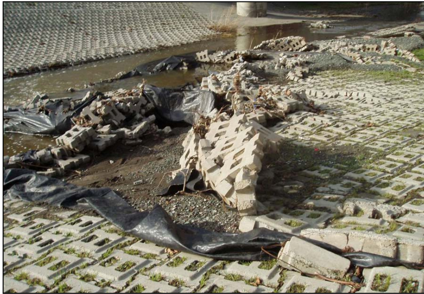
Figure 134. —Insufficient anchorage resulted in uplift of these ACB blocks during flow.
