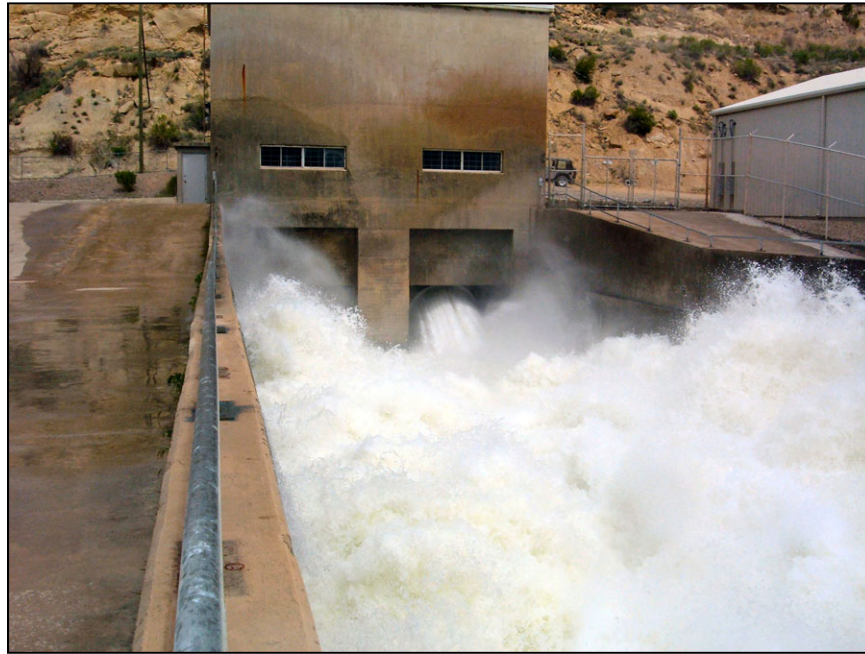
Figure A-55. —Both hollow-jet valves being operated at near full discharge capacity.
