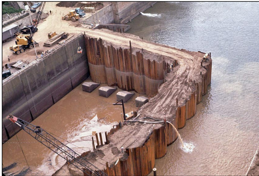
Figure A-38.—Abrasion erosion of stilling basin slab. Note the constructed cellular cofferdam that encloses a portion of the basin.
