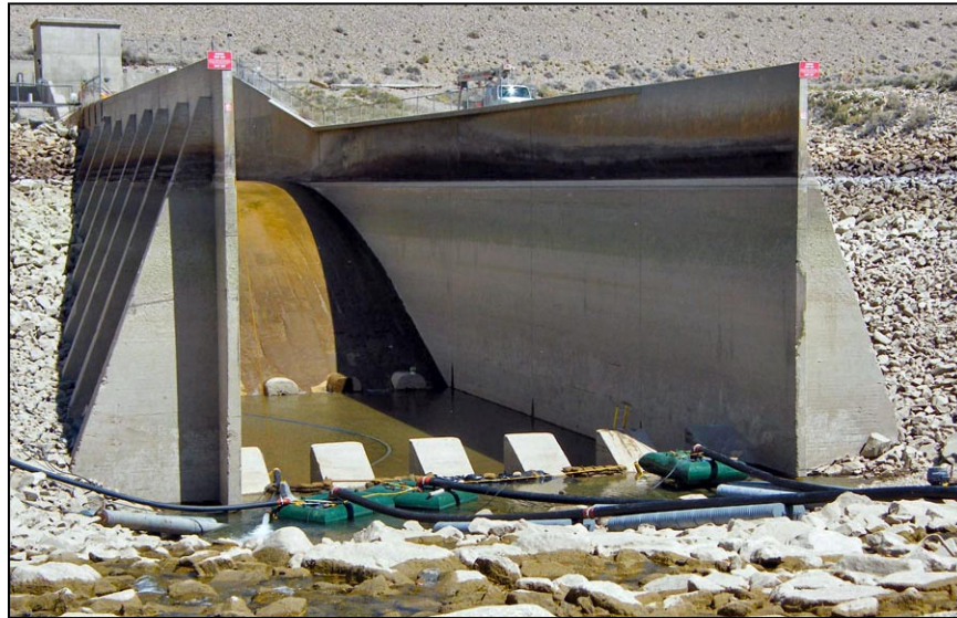
Figure 24. —Type II stilling basin with counterforted walls. The basin has been unwatered for repairs.
