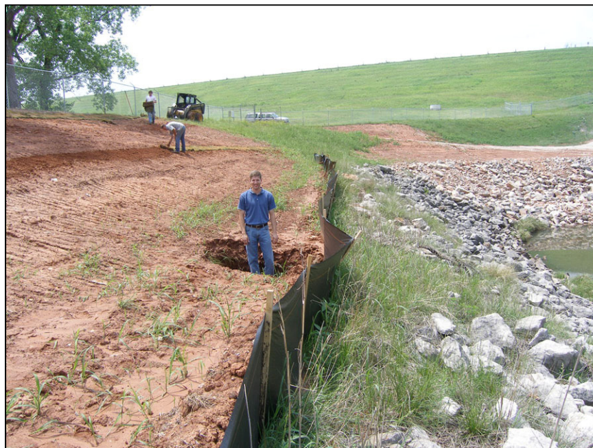
Figure A-66. —After the basin was refilled, a sinkhole approximately 3 feet deep and 3 feet wide appeared on the surface of the bank above the water line.
