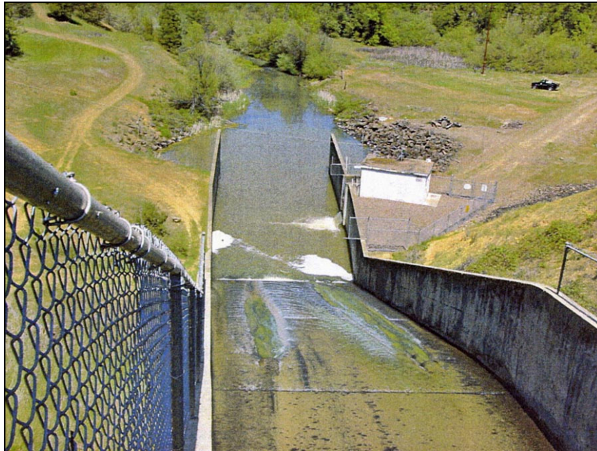
Figure A-1. —Combined spillway and outlet works basin. The sleeve valve is located in the control house on the right side of the basin.
