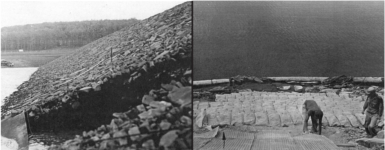
Figure 27: Sinkhole in Upstream Slope of Dam at Waterline (left); Temporary Repaired Sinkhole with Gravel, Geotextile and Sandbags (right)
