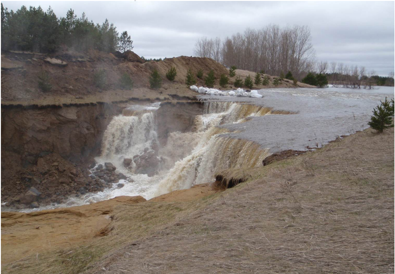
Figure 9: Severe Auxiliary Spillway Erosion
