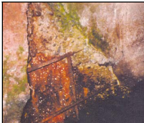
Figure 114. —Spalled concrete and exposed reinforcement in an outlet works conduit.
