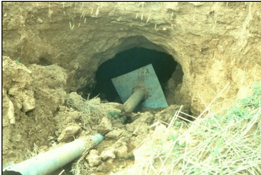
Figure A-2. —Internal erosion failure along a conduit with antiseep collars.
