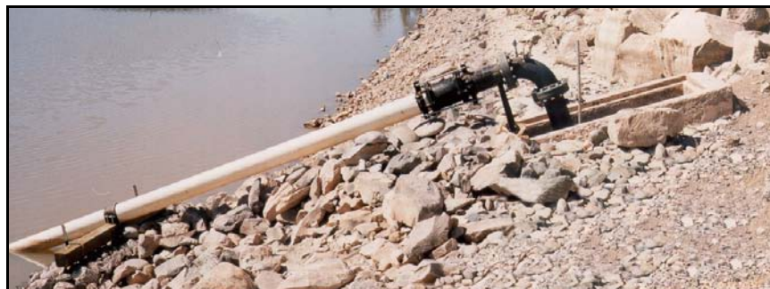
Figure 150. —Siphon used to lower the reservoir water surface through the upper entrance of an outlet works intake structure.
