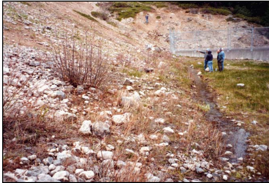
Figure 118. —Visual inspection for seepage on the downstream face of an embankment dam.
