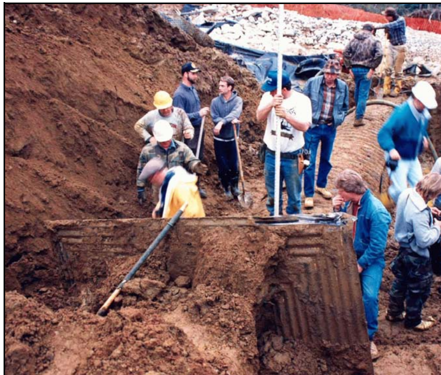
Figure B-8. —Starting at the downstream end of the conduit, two large excavators removed the majority of the earthfill under the watchful eyes of State and local officials, geotechnical engineers, surveyors, lawyers and the pipe manufacture.
