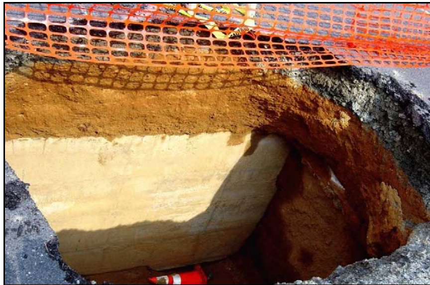
Figure B-27. —The road was closed immediately, and lake level was lowered. However, the sinkhole rapidly enlarged.
