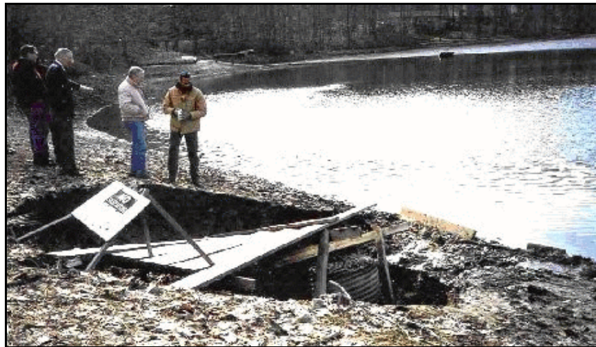
Figure B-67. —When the 35-year old corrugated metal pipe riser collapsed, a large portion of the low hazard embankment dam was washed away. This left a void about 30 feet in diameter and 10 feet deep around the original riser.
