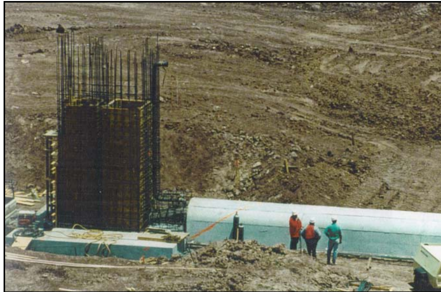
Figure 72. —Special design considerations are required in locations where differential settlement between two structures can occur.
