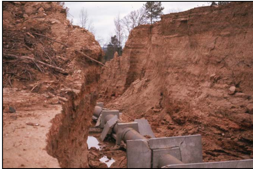
Figure 17. —Failure of an embankment dam following first filling. The failure was attributed to internal erosion because the time required for seepage to develop through the compacted embankment and cause failure was very short. Also, the soils are not the type ordinarily considered susceptible to backward erosion piping. Antiseep collars were not effective in preventing the failure.
