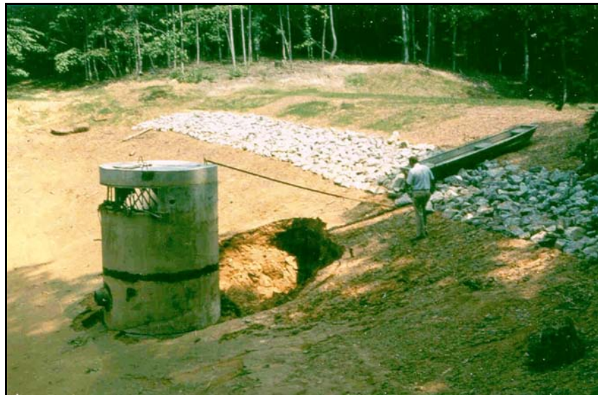
Figure 120. —Sinkhole around a spillway riser. Photo courtesy of Schnabel Engineering.
