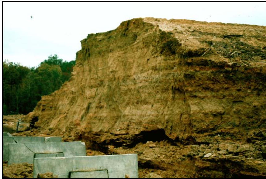
Figure 82. —The failure of this embankment dam located in South Carolina was attributed to hydraulic fracture. The eroded seam located to the right of the conduit may have been the hydraulic fracture that formed and allowed internal erosion and failure of the embankment dam. The embankment was composed of dispersive clays.
