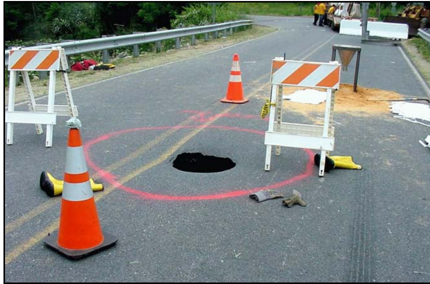
Figure B-26. —Less than 2 years later, an engineer inspecting the bridge over the spillway reported that seepage flow was visible from under the downstream end of the spillway. The seepage flow was clear, and no migration of soils was evident. A few months later, the roadway on the dam crest collapsed, and large quantities of sediment were observed in the pool below the dam.
