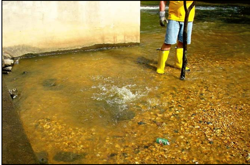
Figure B-28. —Seepage flow at the downstream end of the spillway appeared to be boiling. Attempts to create a sandbag weir around the boil to reduce leakage under the spillway were unsuccessful.
