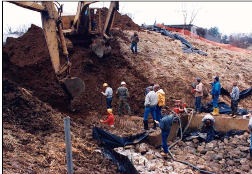
Figure B-7. —The spillway conduit and portions of the embankment soils were carefully removed and documented during a forensic investigation about 2 weeks after the failure.
