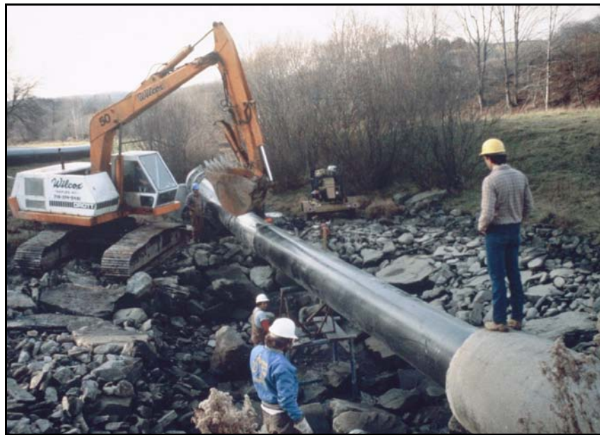
Figure 171. —Insertion of an HDPE slipliner into an existing concrete conduit. A backhoe is being used to assist with slipliner insertion.
