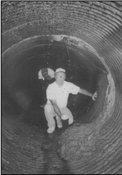
Figure B-36. —A man-entry inspection of this 60-inch CMP noted seepage and extensive loss of embankment soil at two locations.
