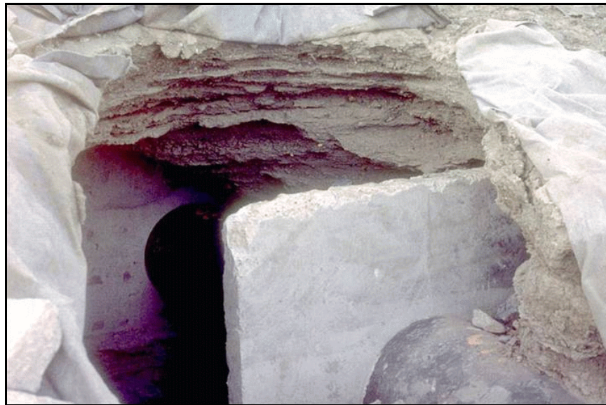
Figure 18. —Antiseep collars were not adequate to prevent the internal erosion failure of this embankment dam. The internal erosion that occurred on first filling of the reservoir occurred in dispersive clay soils that are not susceptible to backward erosion piping.
