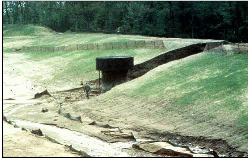
Figure B-50. —Loveton Farms Dam failure as viewed from upstream. Note that the walls of the failure area are nearly vertical. The construction records indicate that a large portion of the embankment dam was placed prior to installation of the CMP.
