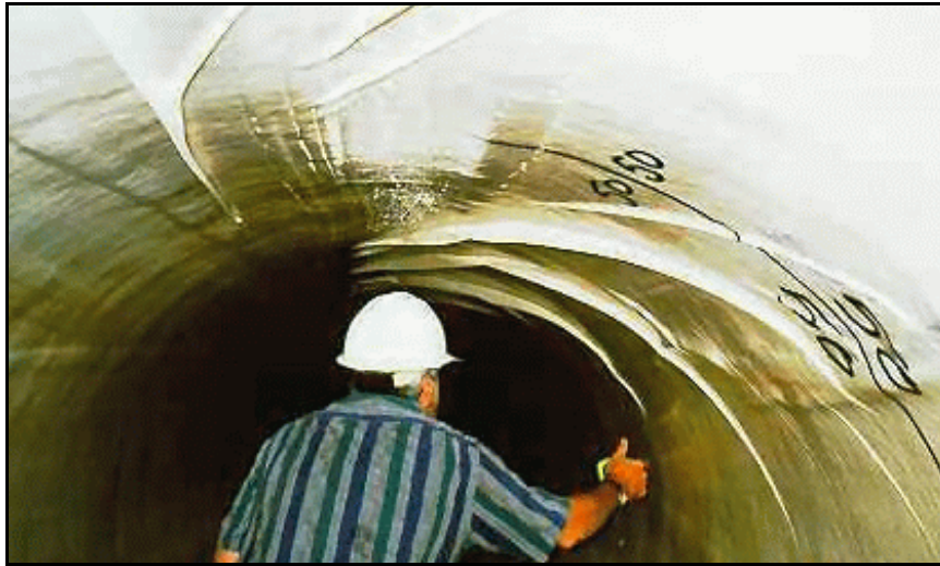
Figure 185. —The calibration hose of this pulled-in-place CIPP developed “fins.” These fins were considered to have an insignificant effect on hydraulic capacity for this particular conduit application and were not removed.
