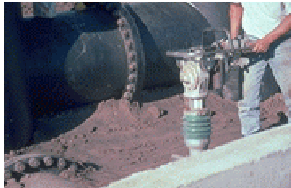
Figure B-4. —Initial construction. Note hand tampers being used to compact earthfill adjacent to outlet conduit.
