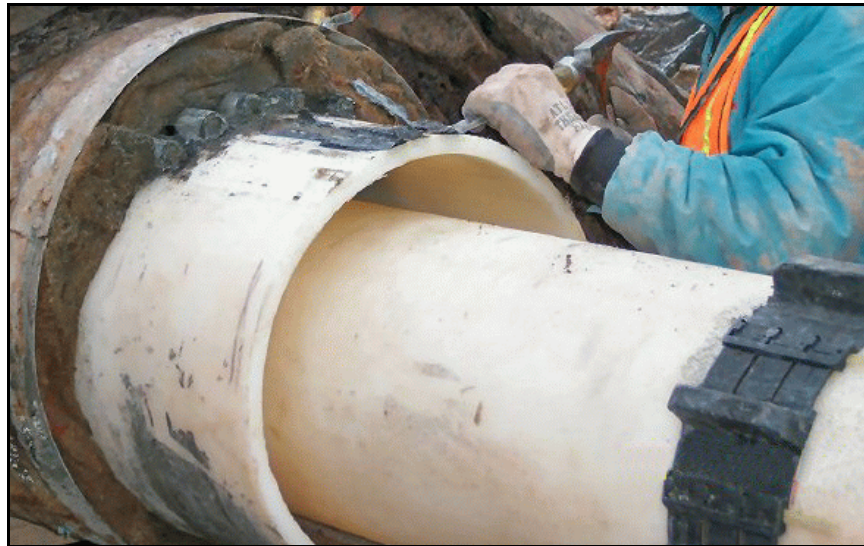
Figure 178. —A 14-inch diameter interior HDPE pipe is being inserted into a 20-inch diameter outside pipe. Intermediate spacers are used to keep the interior HDPE pipe centered and supported. The annulus grouting between the existing CMP and exterior HDPE pipe has been completed.
