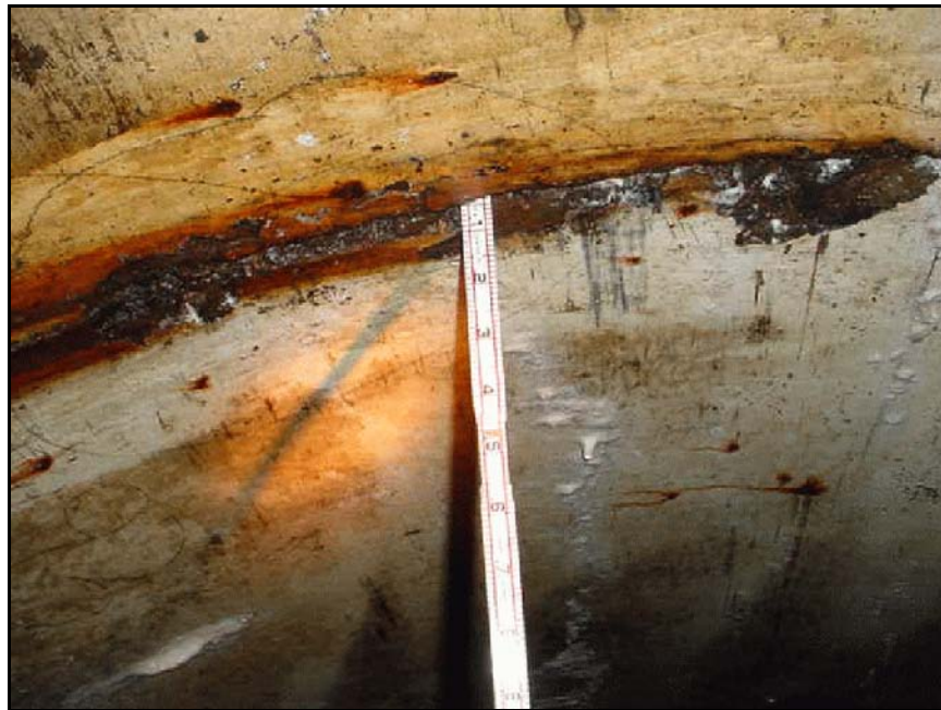
Figure B-23. —Spall at the construction joint located at station 4+93.
