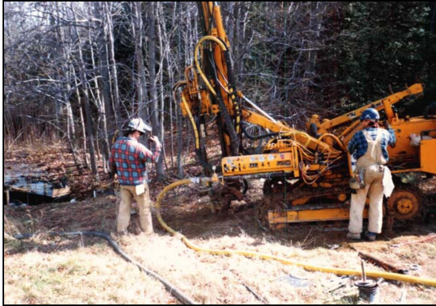
Figure 197. —Abandonment of a conduit by injection of cement grout through holes drilled from the surface of the embankment dam to depths of up to 60 feet.
