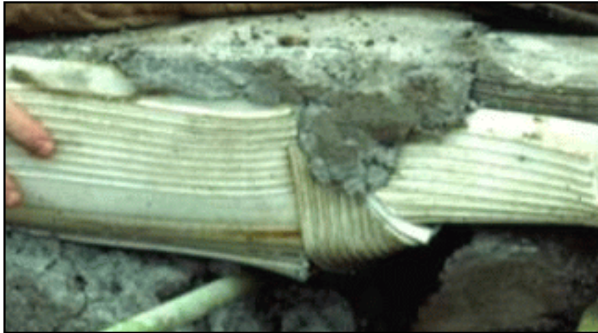
Figure 77. —A poorly secured waterstop moved during concrete placement.
