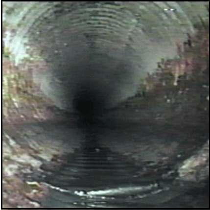
Figure 110. —CMP corrosion within an outlet works conduit.
