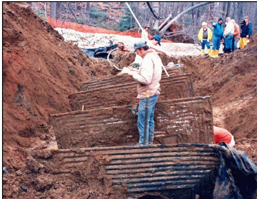
Figure B-11. —Seepage along the sides of the CMP resulted in loss of soil support, causing conduit and joint deformation.
