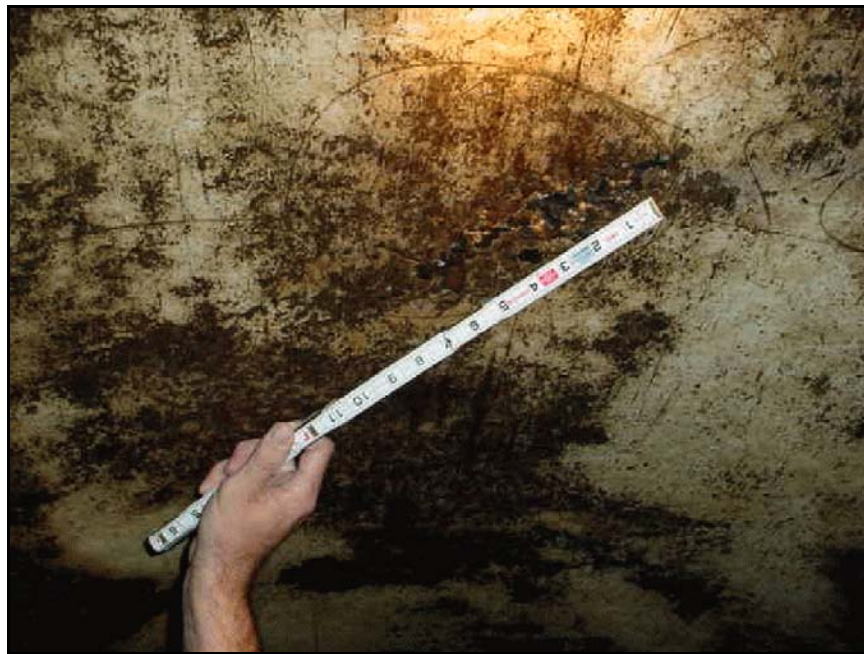
Figure B-21. —Exposed aggregate located at station 11+28.
