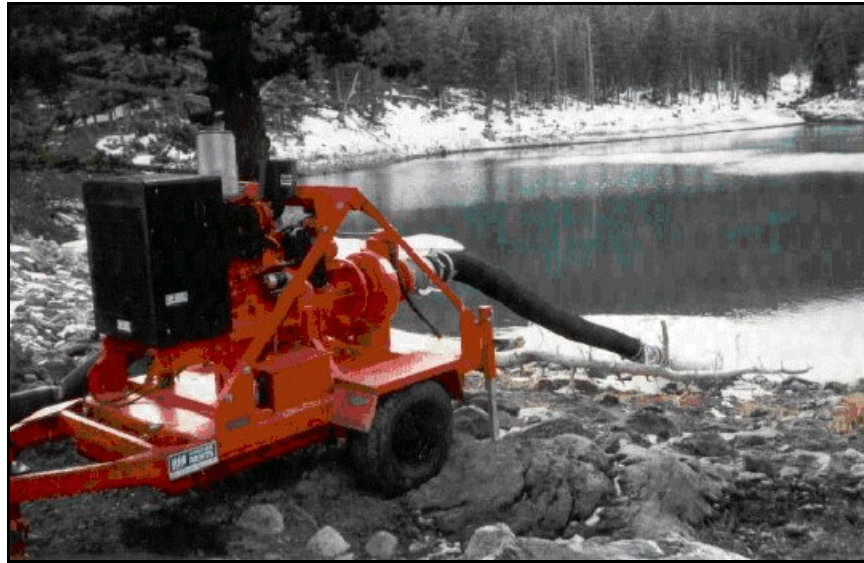
Figure B-17. —Portable pump used to initiate draining of the reservoir.
