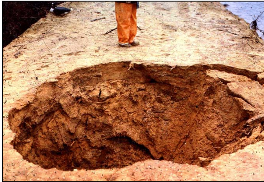
Figure 147. —Sinkhole over a spillway conduit.
