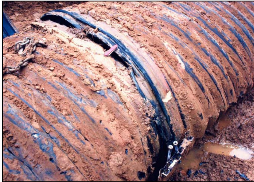
Figure B-9. —When the “hugger band” at the most downstream conduit joint was removed, the o-ring gasket was found to have been displaced. In addition, debris from the pool was found under the band, indicating that water may have flowed unrestricted along the outside of the conduit from the pool and into the joint.
