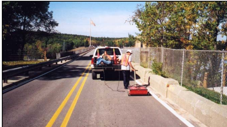
Figure 142. —Conducting a ground-penetrating radar survey across dam crest to locate voids beneath roadway and spillway. Photo courtesy Schnabel Engineering.
