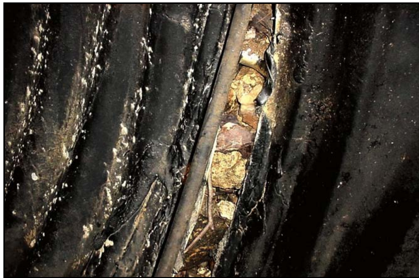
Figure B-52. —The failed embankment dam was repaired with a new 78-in diameter CMP spillway. However, soon after reconstruction, this failed joint was discovered at the upstream end of the pipe near the riser. A large void was also observed in the adjacent embankment fill. Note the o-ring gasket has been displaced from the joint.
