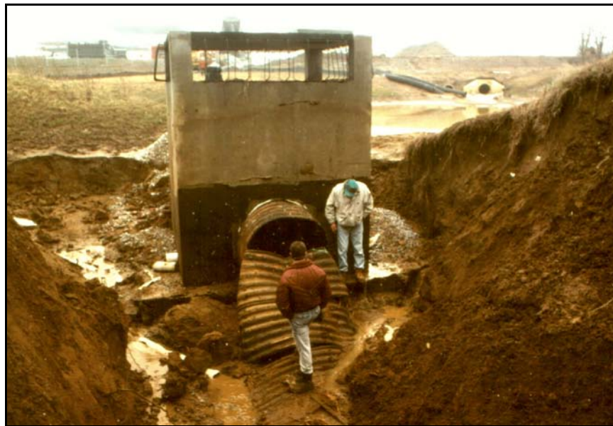
Figure B-5. —The upstream section of the 54-inch diameter CMP spillway conduit completely collapsed when the water level reached the elevation of the weirs on the inlet structure. Site personnel reported a “vortex” in the pool adjacent to the structure shortly before collapse.
