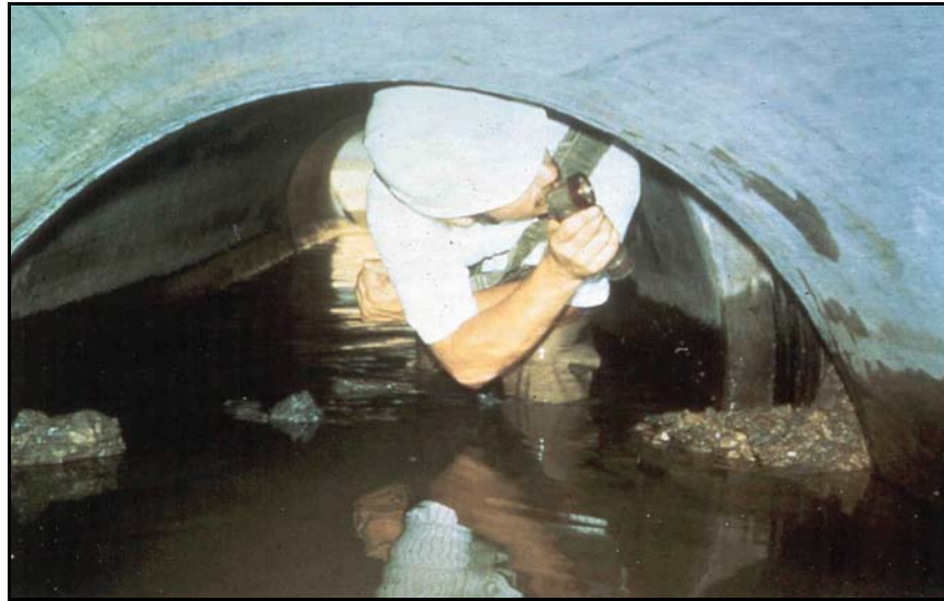
Figure B-49. —The pipe joints separated when foundation movement occurred during construction of the embankment dam.
