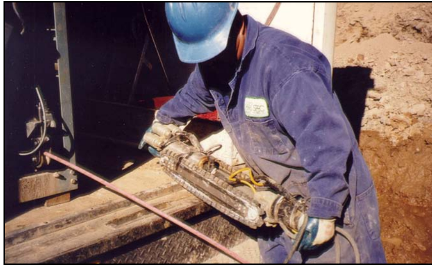
Figure 130. —Most CCTV inspection equipment is portable and can be carried to conduit access locations.
