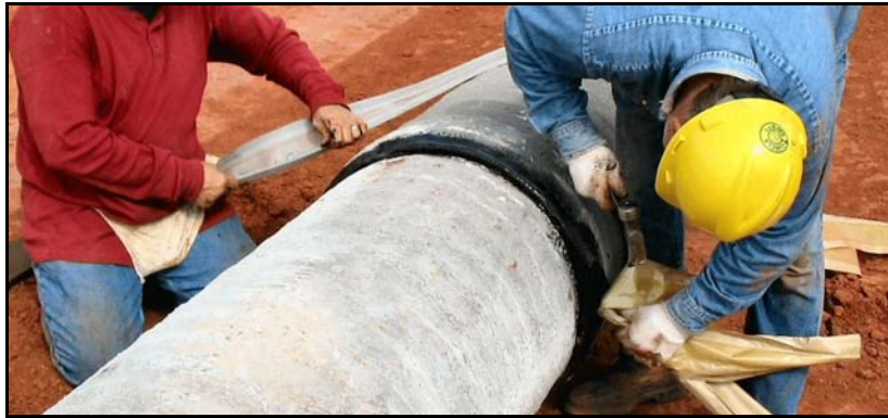
Figure 80. —Mastic being applied to exterior annular joint space of precast concrete pipe.
