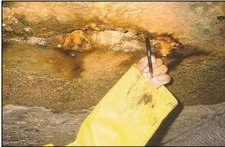
Figure 194. —Evaluate the extent of the damage.
