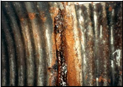
Figure 112. —CMP corrosion within an outlet works conduit caused by a leaking pipe joint.
