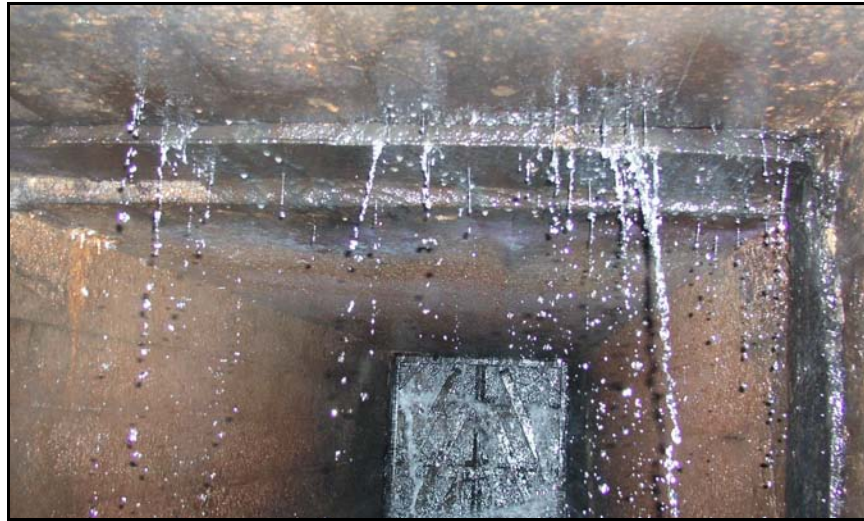
Figure 70. —Water seeping through a joint in an outlet works conduit. The joint has experienced differential settlement. This joint had no longitudinal reinforcement extending across the joint. The mortar joint filling has cracked and deteriorated.
