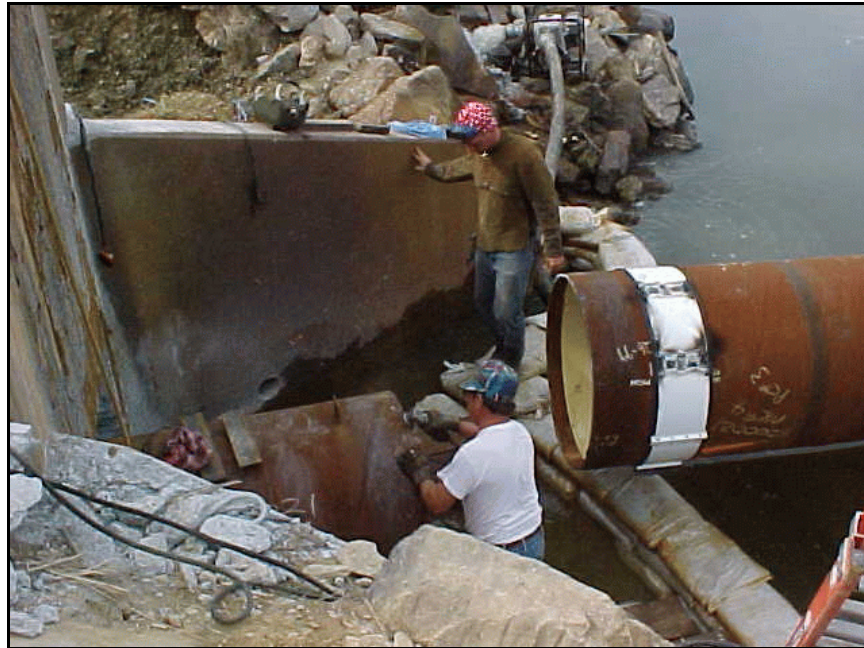
Figure 180. —The Lake Linganore Dam outlet works consists of a 48-in diameter RCP conduit with a sluice gate located at the downstream end, which places the conduit under full reservoir head at all times. Concern about the integrity of the RCP joints led to installation of a steel slipliner when the inoperable sluice gate was replaced.
