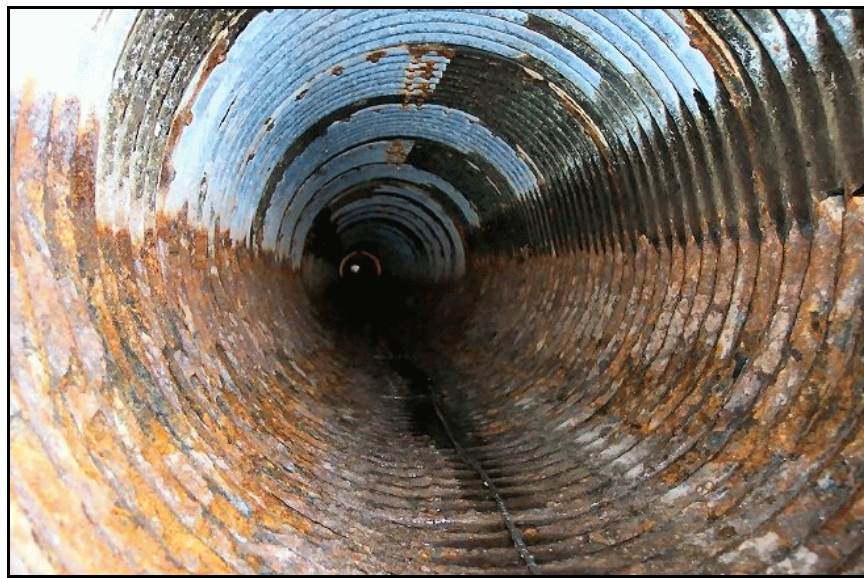
Figure 127. —Corrosion within a 24-inch-diameter CMP outlet works conduit.
