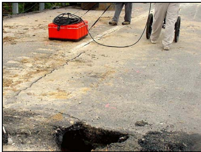
Figure B-31. —Ground penetrating radar identified the location of voids along the CMP.
