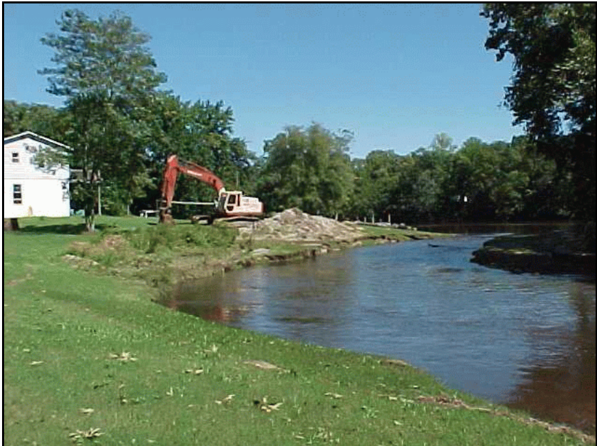
Figure 156.—The owner of this embankment dam excavated a channel around the dam to prevent its overtopping during a hurricane.
