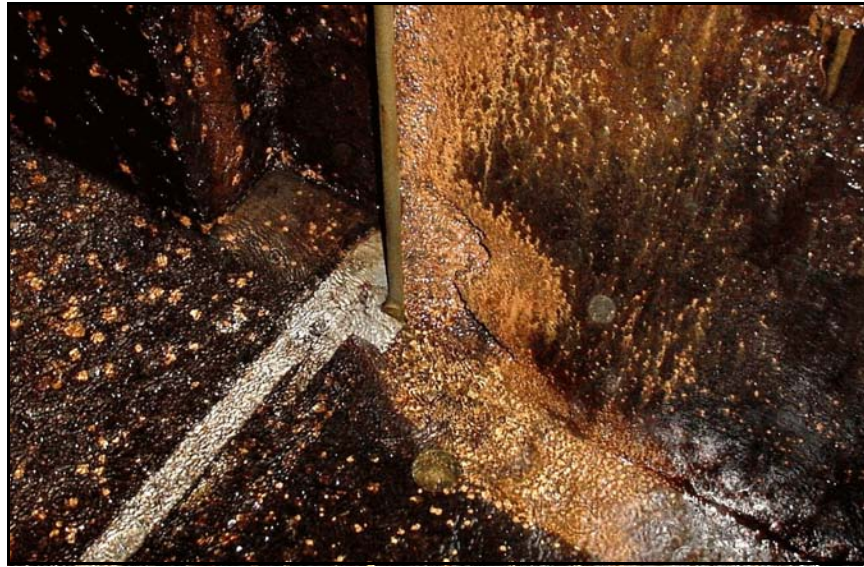
Figure 108. —Cavitation damage to the cast-iron lining of a conduit immediately downstream of a slide gate, caused by high velocity flow.
