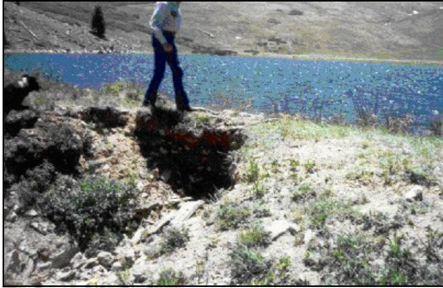
Figure B-37. —Erosion scarp on downstream slope of the embankment dam at the location of the overtopping of the dam crest.
