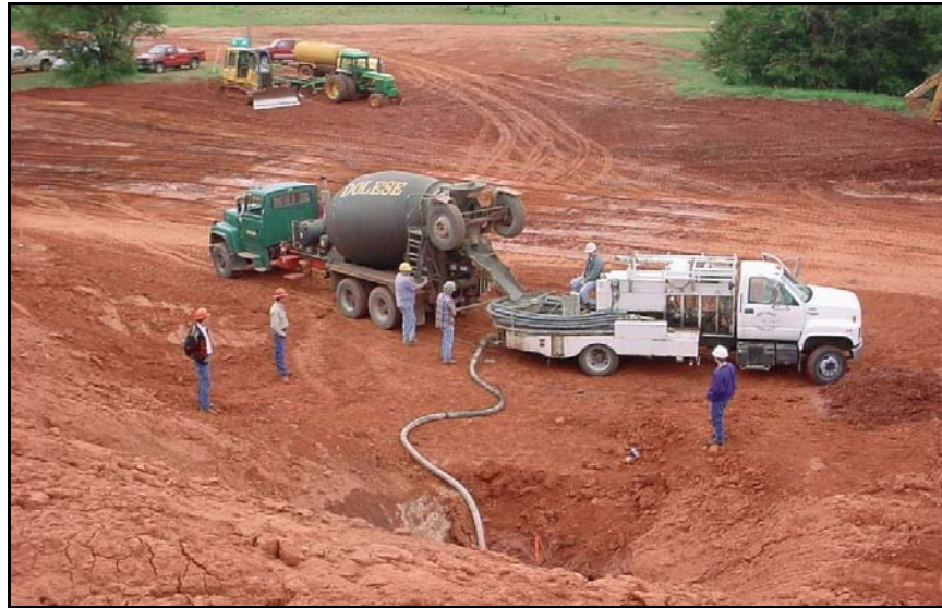
Figure 199. —Grout is delivered to the site and is pumped into the conduit being abandoned.
