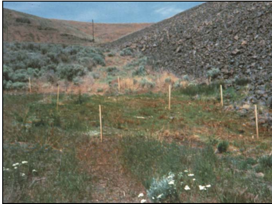
Figure 137. —The perimeter of a wet area at the downstream toe of an embankment dam located with wooden stakes.
