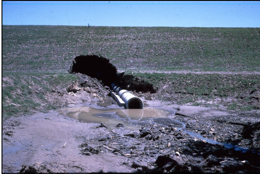
Figure 104. —Failure of an embankment dam due to internal erosion of hydraulic fracture cracks upon first filling of the reservoir.
