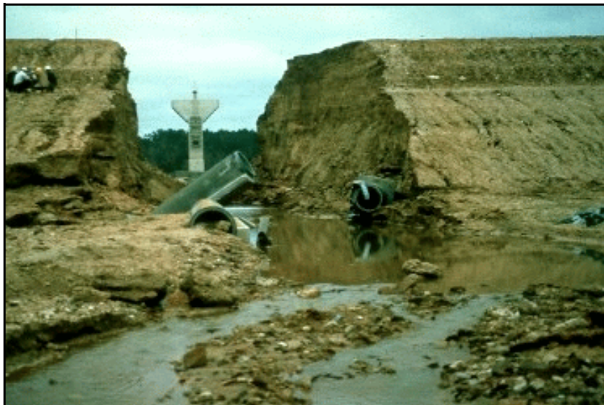
Figure 85. —This embankment dam constructed with dispersive clays failed on first filling of the dam.
