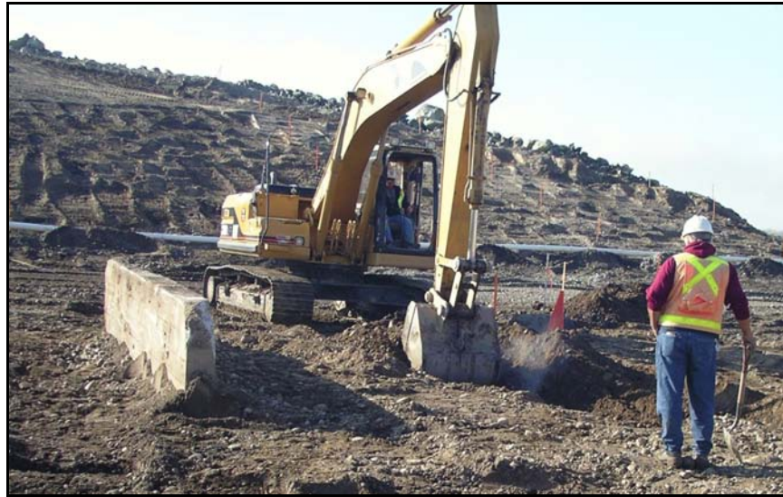
Figure 135. —An outlet works conduit is being excavated during a forensic investigation. The top of an antiseep collar is exposed on the left side of the figure.
