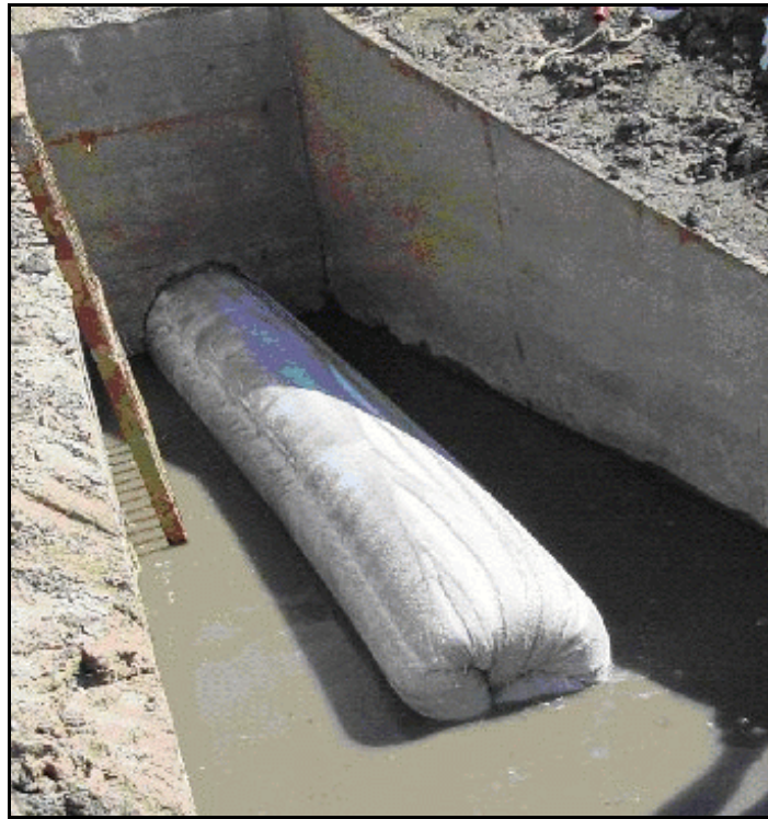
Figure 26. —CIPP liner exiting from an existing conduit via the hydrostatic inversion method.
