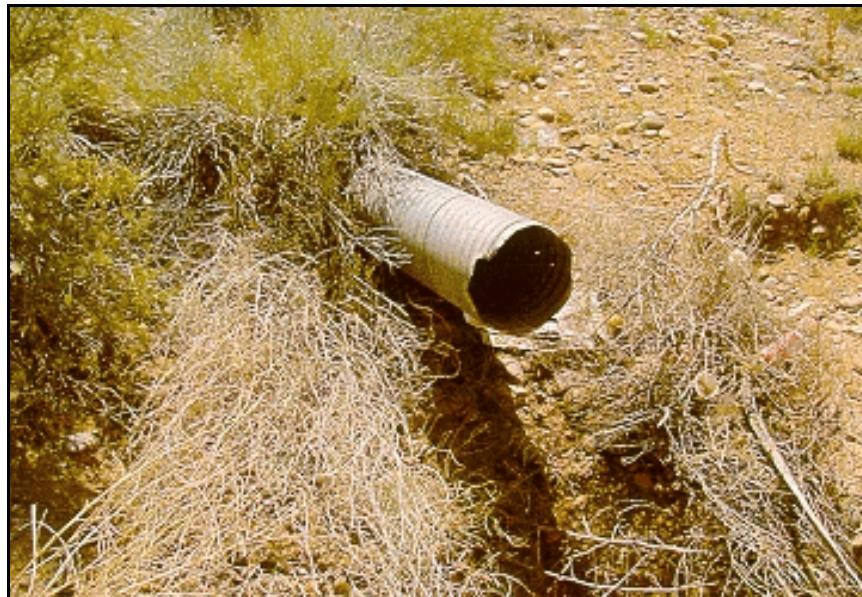
Figure 45. —No terminal structure or erosion protection exists for this outlet works. The embankment around the exit portal has experienced significant erosion.
