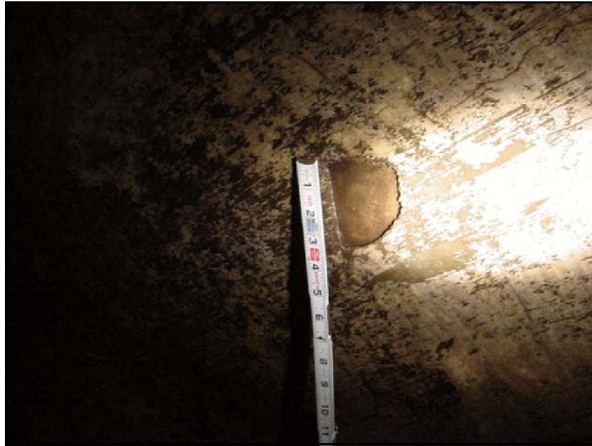
Figure B-22. —Popout located at station 10+79.
