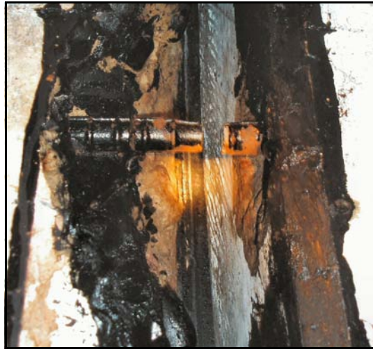
Figure 63. —Longitudinal reinforcement across a conduit joint experienced tensile failure caused by lateral spreading of the embankment dam.
