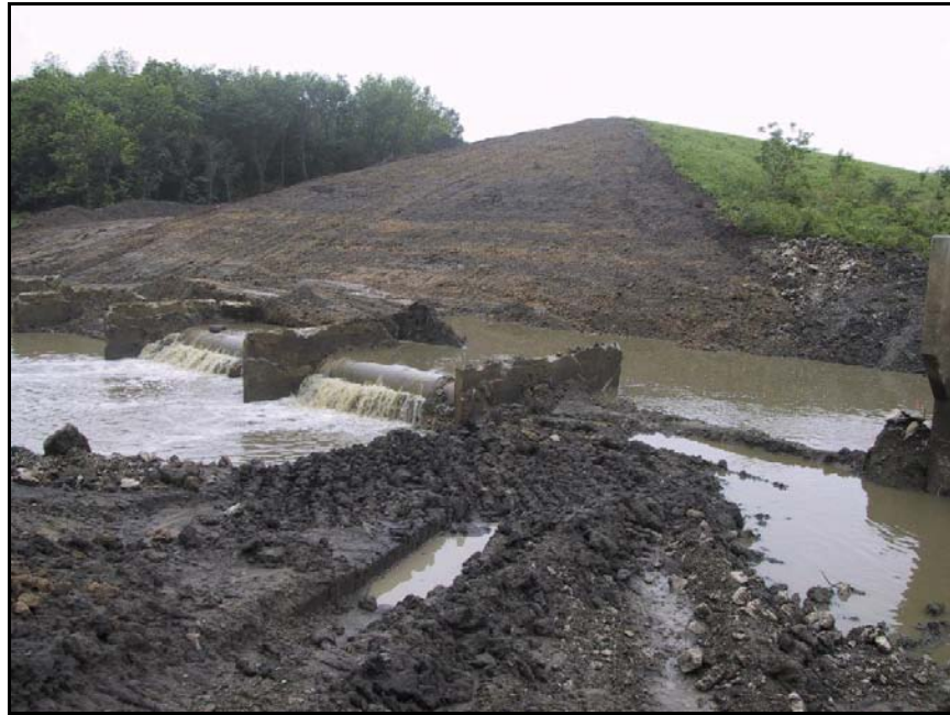
Figure 188. —During the removal of this outlet works conduit a flood occurred. No stream diversion or cofferdam was used at this site.
