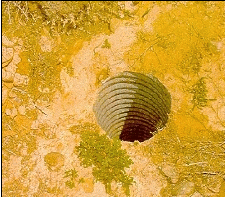
Figure 44. —No intake structure exists for this outlet works. This conduit is prone to plugging with trash and debris.
