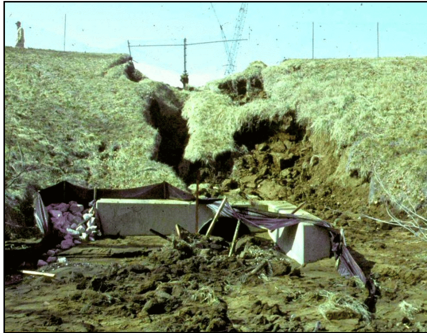
Figure B-6. —The downstream section of the CMP spillway remained partially intact, but deep troughs were visible directly above each side of the conduit.
