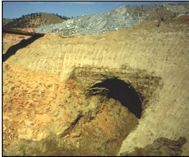
Figure 149. —Incipient sinkhole in an embankment dam. Eventually, the continued removal of the soil at the bottom of the cavern would have caused the roof to migrate to the surface of the embankment dam.
