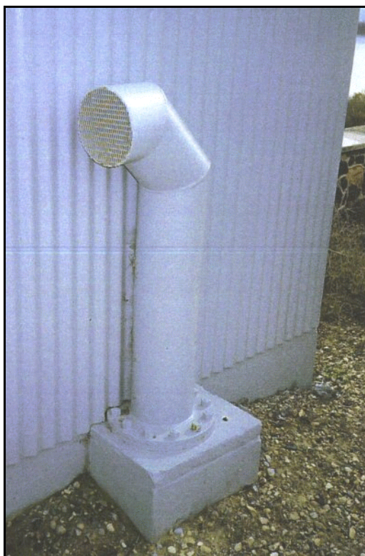
Figure 32. —An air vent is required in closed conduits downstream from the controlling gate or valve to prevent collapse or the formation of low air pressures.
