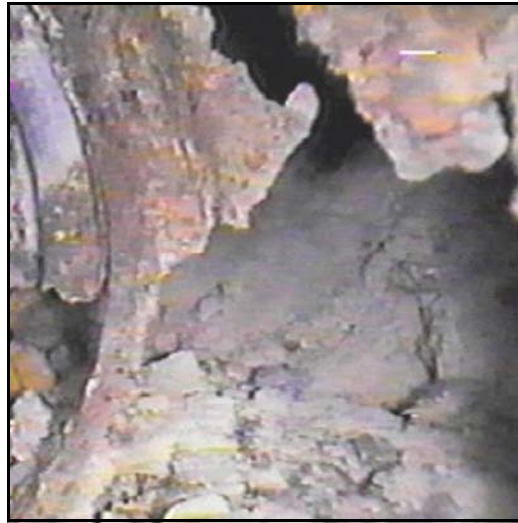
Figure 109. —Corrosion has completely destroyed this CMP spillway conduit. Backfill materials that surrounded the conduit have been eroded by flow within the conduit.
