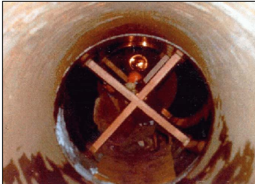
Figure B-34. —Installing the steel pipe slipliner within the existing outlet works conduit.
