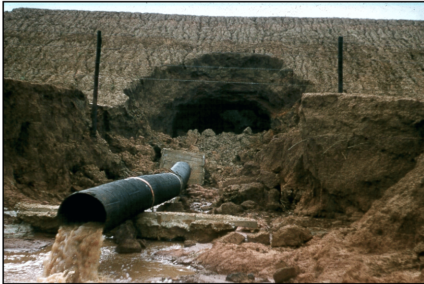
Figure 84. —An embankment dam in Mississippi constructed of dispersive clay soil, failed on first filling with low reservoir level. Failure was likely caused by cracks from differential settlement, hydraulic fracture, or poor compaction about the outlet works conduit. This embankment dam had no filter.
