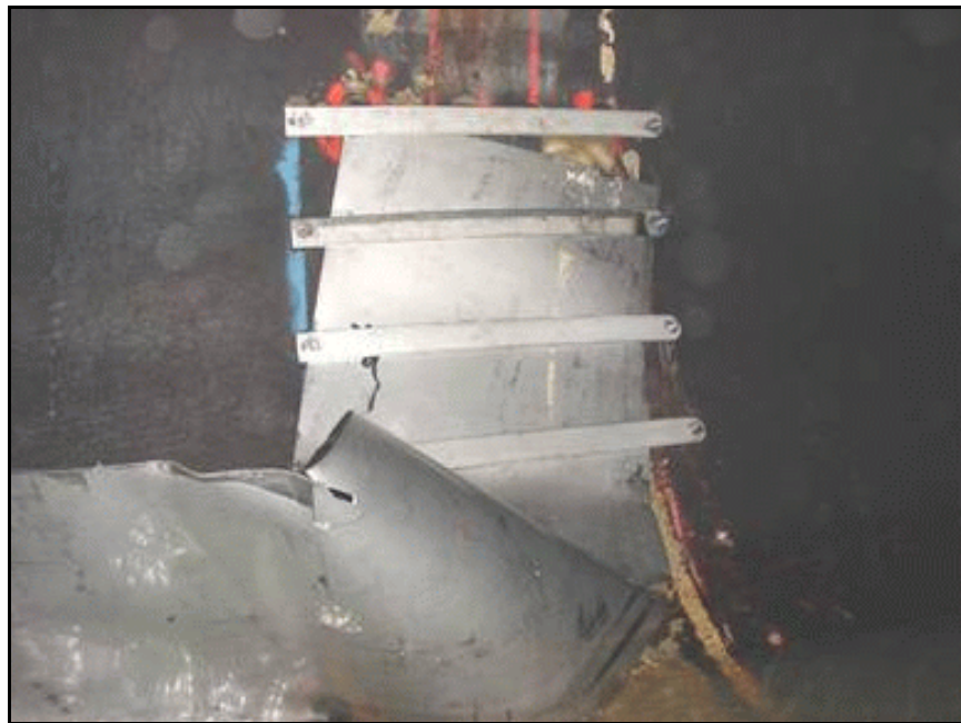
Figure B-15. —Damaged metal plate.
