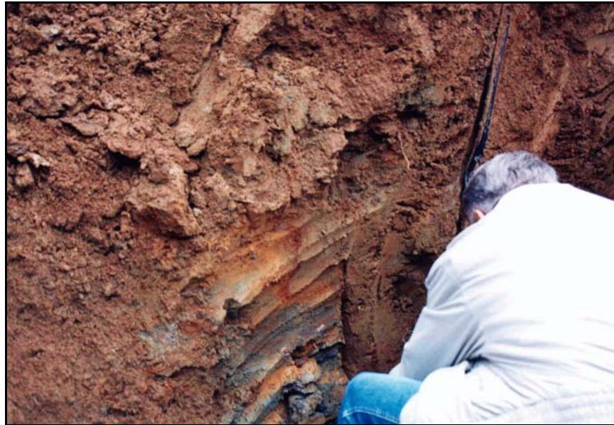
Figure B-10. —The presence of undisturbed foundation soils confirmed that the conduit was placed in a trench with nearly vertical sides, making it difficult to obtain good compaction of the fill soils under and along the CMP and around the antiseep collars.
