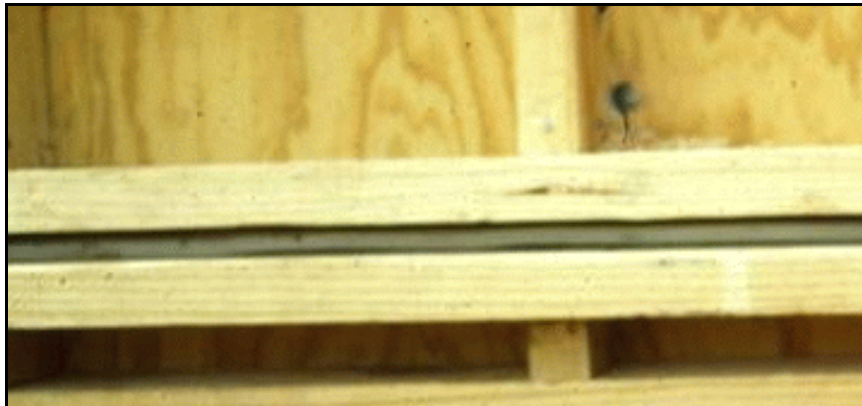
Figure 78. —Waterstop held firmly in place by use of a specially cut slot in the form.
