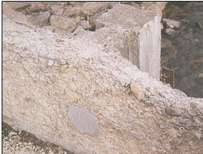
Figure 106. —Concrete deterioration from freezing and thawing.
