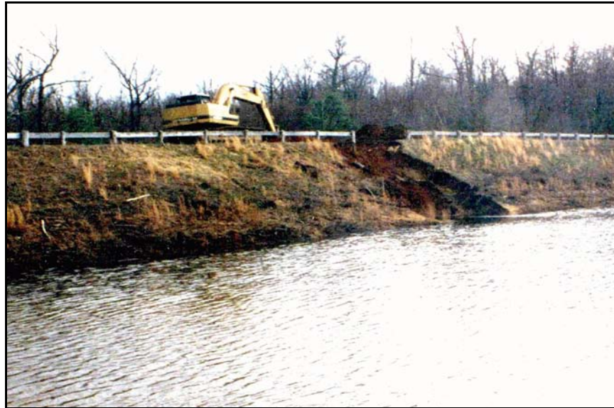
Figure 157. —A controlled breach of an embankment dam begins after the 45-year old CMP spillway conduit collapsed and the lake level began to rise.
