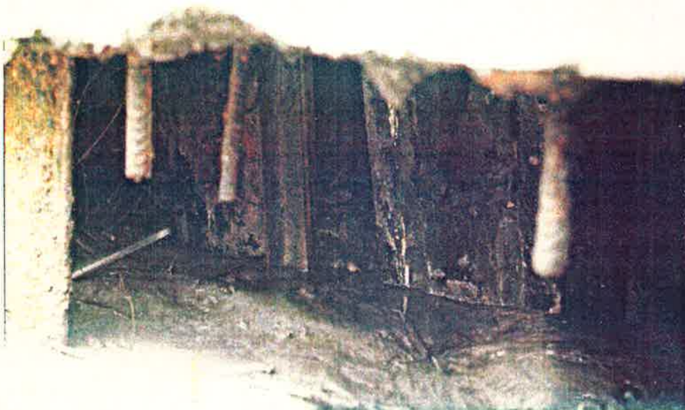
Photo No. 11 7-2-84 The Upper and Lower Photos Show Exposed Rebar and Cavitation Beneath the Structure
