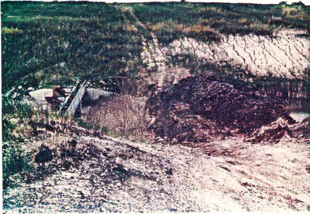
Photo No. 23 7-3-84 The Upper and Lower Photos, Looking West, Show the Project Upon Completion of the 1st Phase of Repair
