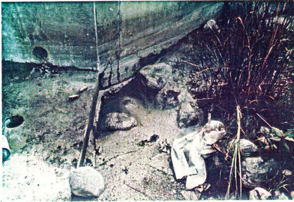
Photo No. 27 8-2-84 Close-up View Showing Inspection Hole On East Wall and an Eroded Area Near The East Downstream Wingwall
