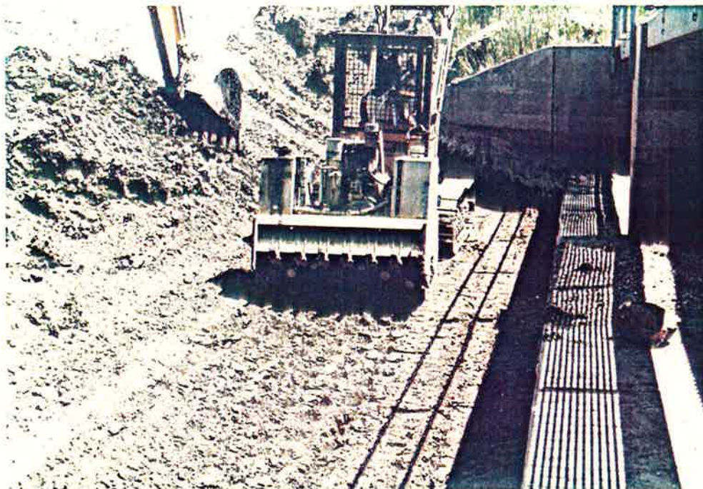
Photo No. 16 - Compaction & Excavation Operations Case 350 Crawler Tractor Pulling Ray Go Compactor Note the Bucket of the Excavator - At this Point, We Had Begun to Excavate Into the Existing Cofferdam to Enlarge Our Impervious Cutoff Area.
