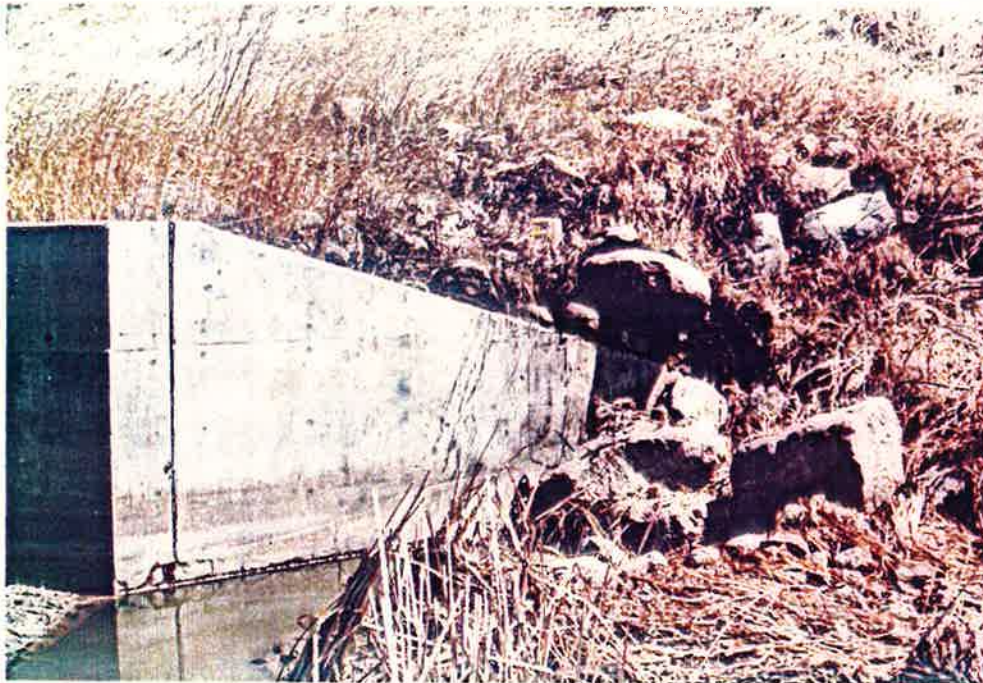
Photo J - Close-up View of East Downstream Wingwall Note the Area that has Slumped Due to Seepage Adjacent to the Wingwall May 8, 1984
