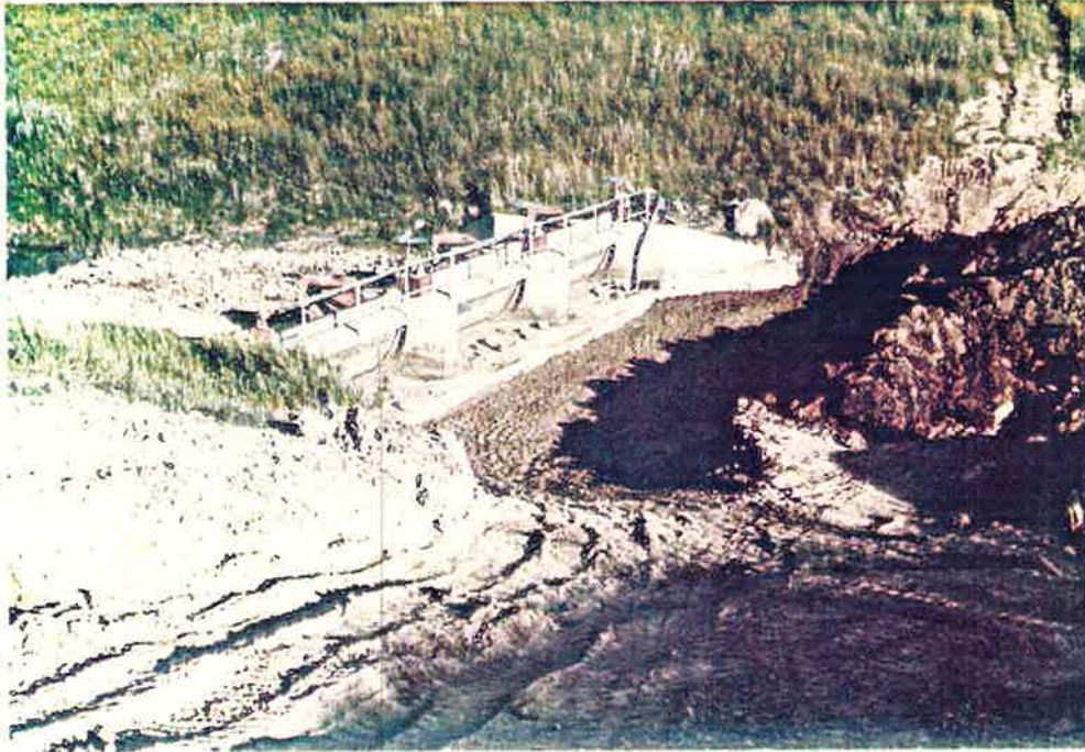
Photo No. 19 - Tuesday 8:00 p.m. 7-3-84 View of Structure & Completed Earthen Backfill Note the Dry Condition of Entire Area After Completing Backfill Operations the Previous Day
