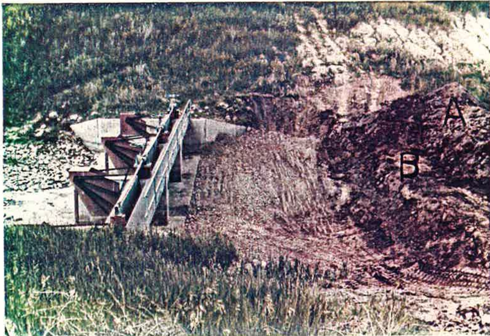
Photo No. 22 7-3-84 View of Structure, Clay Core and Cofferdam The Upper Portion (A) of the Cofferdam Represents the Material that was Excavated on July 2, 1984, to Enlarge the Claycore. The Lower Portion (B) Represents The Original Height of the Cofferdam as First Built
