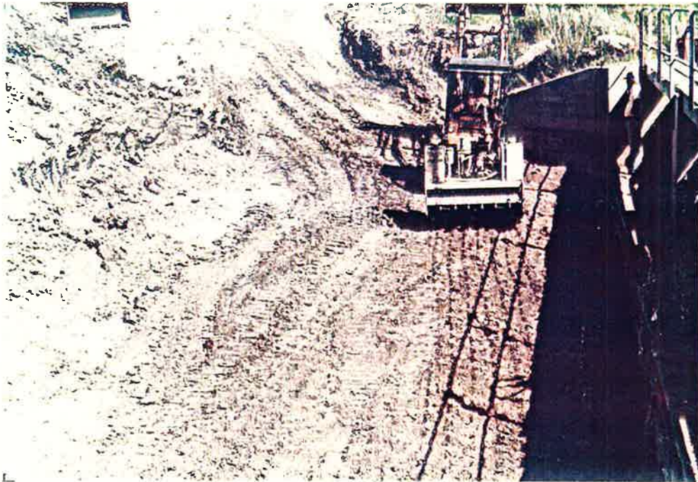
Photo No. 18 - View of Compaction Operations Note the Entry and Exit Ramp to the Left of Equipment 7-2-84
