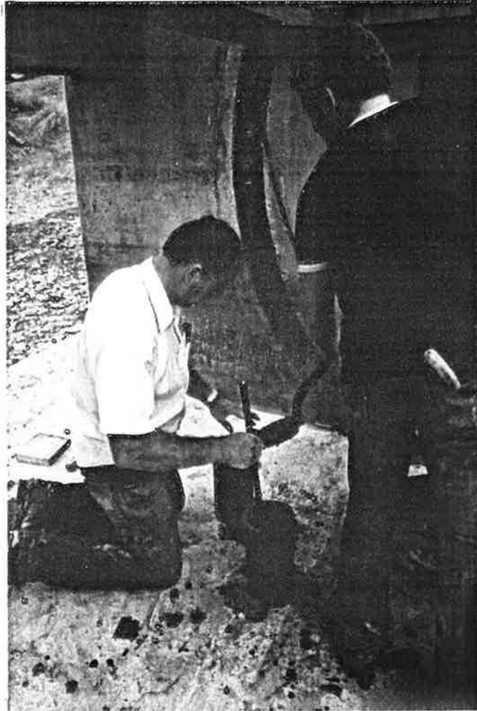
Photo No. 32 8-3-84 Making Concrete Specimens in the Field, in Accordance With ASTM Designation C31. The Compressive Strength of the Molded Concrete Cylinders Were Later Determined by Twin City Testing and Engineering Laboratory, Inc., Grand Forks, North Dakota
