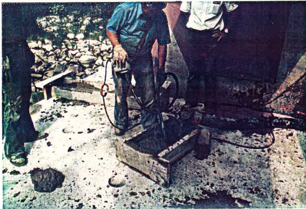
Photo No. 30 8-3-84 View Showing Concrete Being Vibrated Down into the Structural Foundation
