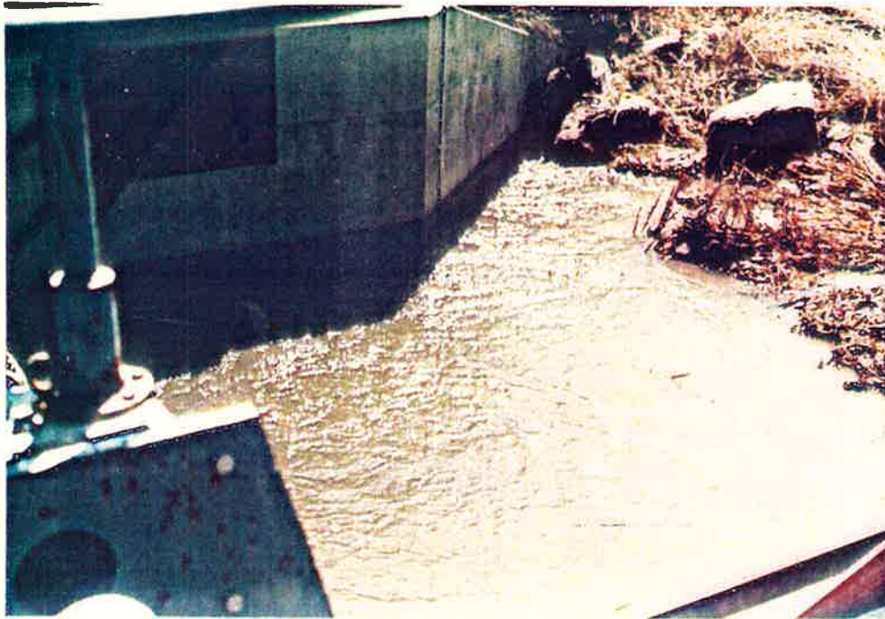
Photo I - View of the East Downstream Wingwall Water was Reportedly Flowing Along the Soil Side of the Wingwall and Emerging in the downstream Pool May 2, 1984
