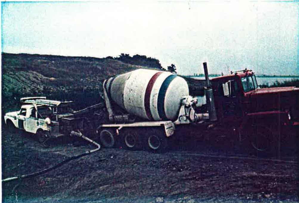
Photo No. 28 8-3-84 Concrete Pumping Operations The Concrete is Delivered to the Site by a Truck Mixer, Discharged by Chute into a Pumper, and Then Pumped by Hose into Holes Previously Drilled on the Structural Floor
