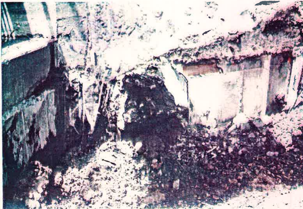
Photo No. 9 - 7-2-84 The Upper and Lower Photos Show Further Evidence of Poor Workmanship and Improper Construction Methods. Note the Large Chunk of Concrete Protruding Beyond the Face of the West Upstream Wingwall and the Wood Framework Left Inplace
