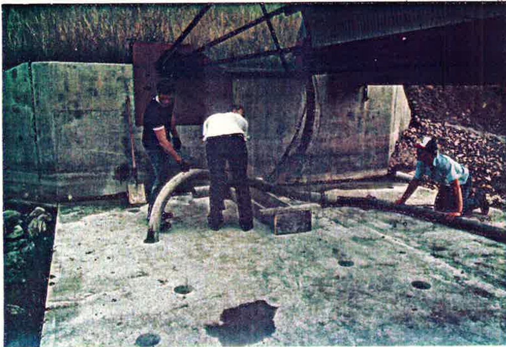
Photo No. 29 8-3-84 Concrete Pumping Operations Close-Up View of Concrete Being Pumped into the Structural Foundation Note the Drilled Holes on the Floor An Attempt Was Made to Pump Concrete into Each Hole
