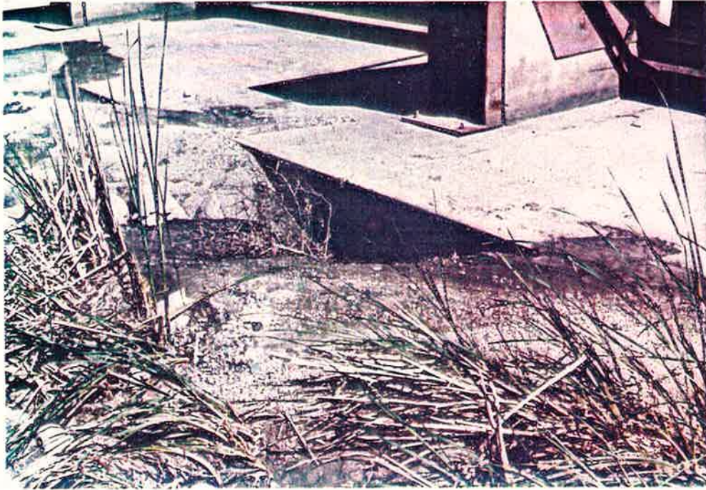
Photo No. 1 - Sink Hole Downstream of Structure 6-27-84
