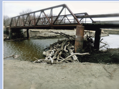
The flood of 2011 caused significant problems such as large snags at river crossings.
