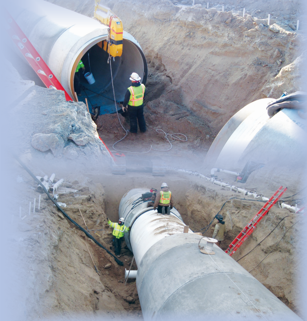
The transition sections (above) and final connecting section (below) of the outlet pipeline are installed by Garvey Construction crew members.
