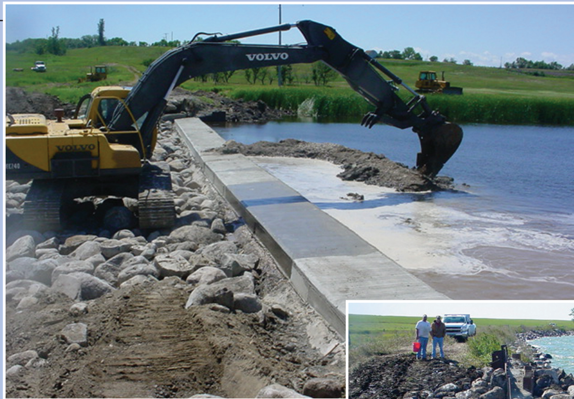
The new concrete cap and rock riprap fish passage at Sheyenne Dam.
