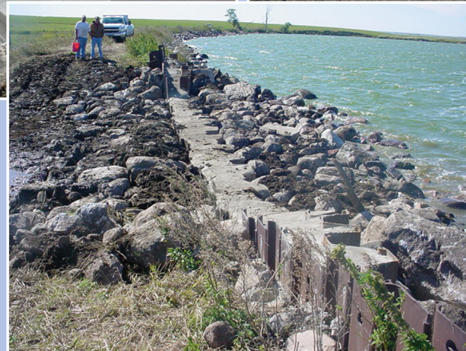
At the Green Lake project, concrete was poured between two sections of sheet pile and rock protection was installed on both the upstream and downstream sides of the structure.
