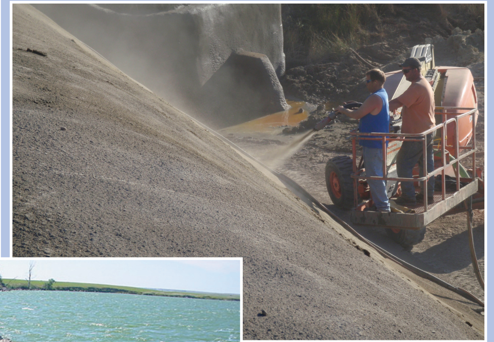
Commission construction crew members Dan Bahm and John Edwards resurface Odland Dam with gunite.
