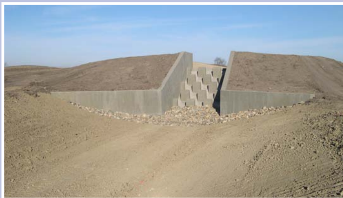
Drop Structures: Both drop structures are completed. One involves a 15-foot drop, the other is slightly larger at 17 feet of drop.
