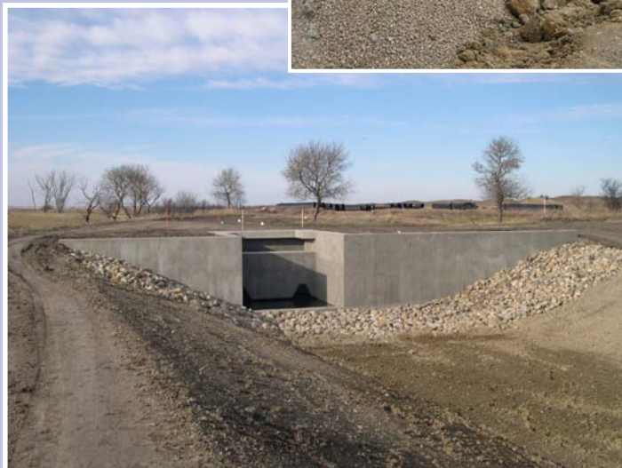
Transitions: There are two transition structures included in the outlet design. They mark the areas where pipeline connects with canal. Transition #2 is complete, and transition #1 is substantially complete, with only minor construction and clean-up remaining.
